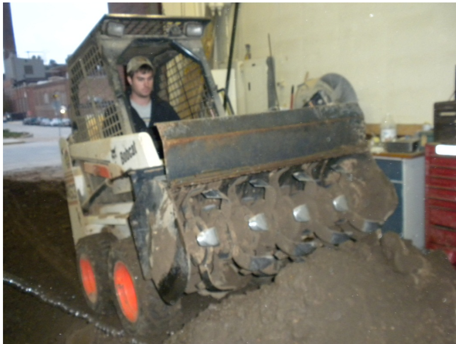
Figure 3.20 Preparation of soil for uniform moisture content prior to placement and compaction.
