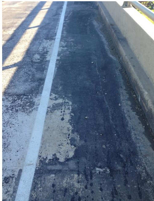
Figure 40. Example of a worn off spot of asphalt emulsion showing concrete underneath
