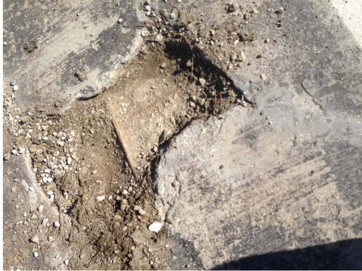
Figure 38. Concrete popout revealing rebar
