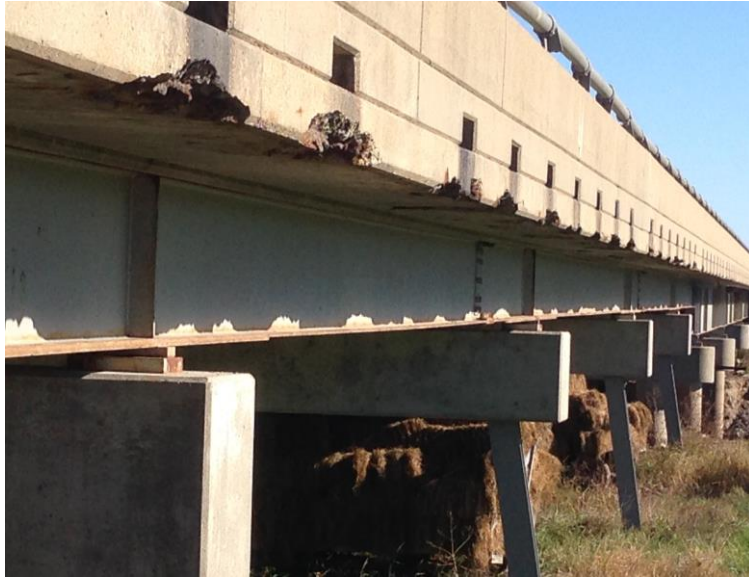
Figure 35. Numerous holes shown corroding throughout the span of the bridge
