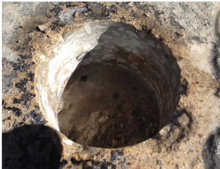
Figures 52. Core popped out with diagonal entry and exit of steel reinforcement
