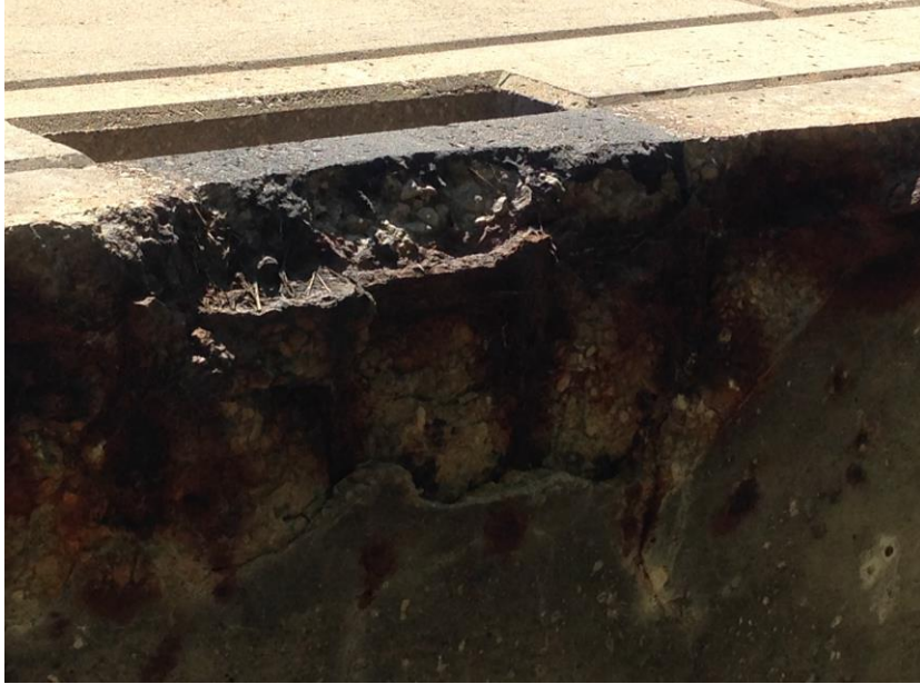
Figure 37. Rebar spacing shown underneath the bridge in corroded section
