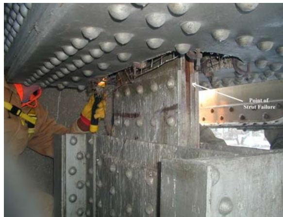
Figure 1.4 Point of Strut Failure
