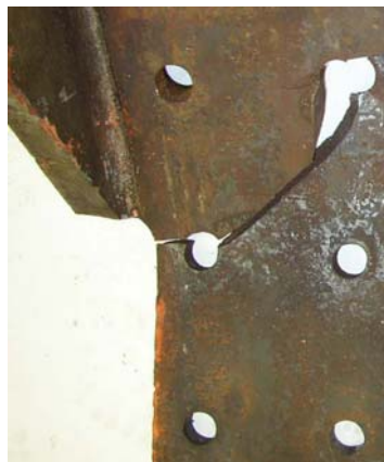
Figure 8.12 Actual Crack Propagation Pattern
