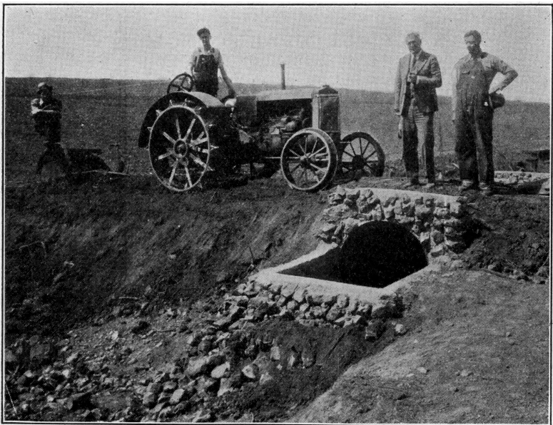
Inlet view of a newly constructed soil saving dam on the farm of John T. Rosewicz, Barry county.
