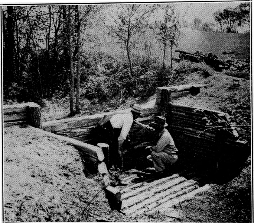
Hedge log dam and spillway in ditch on farm of W. A. Hargadine in Linn county.
