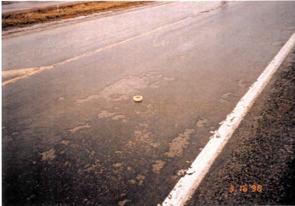
Photo #1: Wear and loss of seal on the surface. The roll of masking tape can be seen for size reference. March 16, 1998; District 4, Lafayette County Route 24
