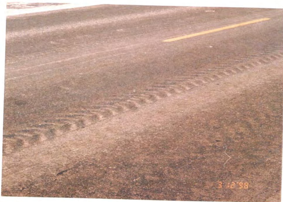
Photo #2: Grader tire marks in the surface. March 12, 1998; District 3, Audrain County Route 22
