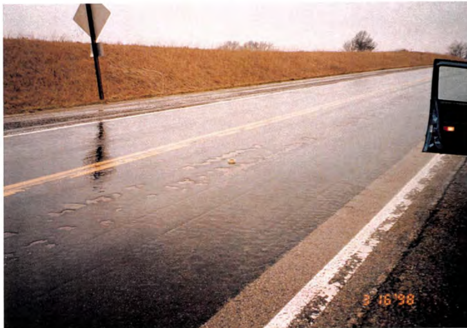
Photo #2: More wear and loss of seal. The masking tape can be seen for size reference. In the vicinity of the car door, it can be seen where the seal was applied in such a fashion that the entire width of the lane was not covered. March 16, 1998; District 4, Lafayette County Route 24
