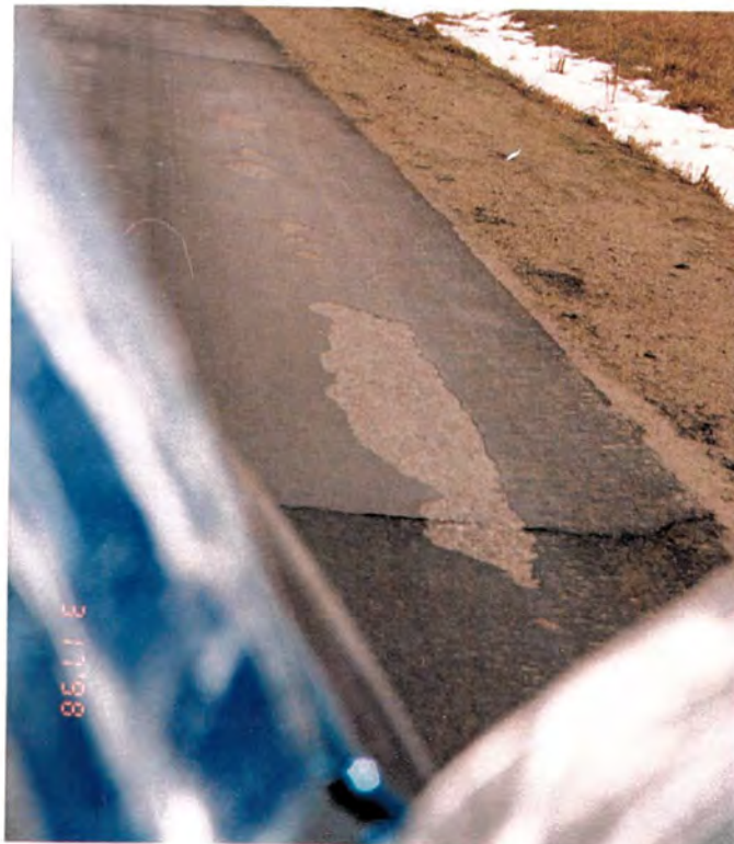
Photo #2: A loss of seal in the wheelpath. March 17, 1998; District 1, Buchanan County Route JJ
