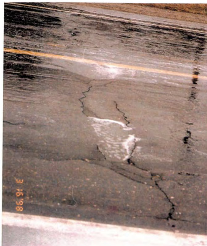
Photo #2: Ponding on the driving surface. March 16, 1998; District 2, Chariton County Route 24
