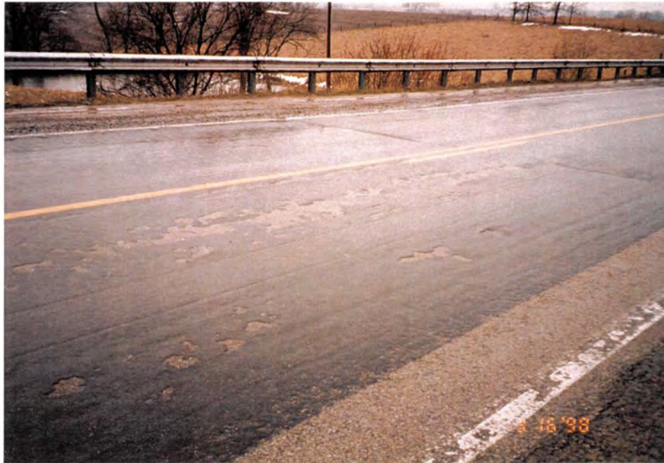
Photo #5: Still more wear and loss of seal. March 16, 1998; District 4, Lafayette County Route 24
