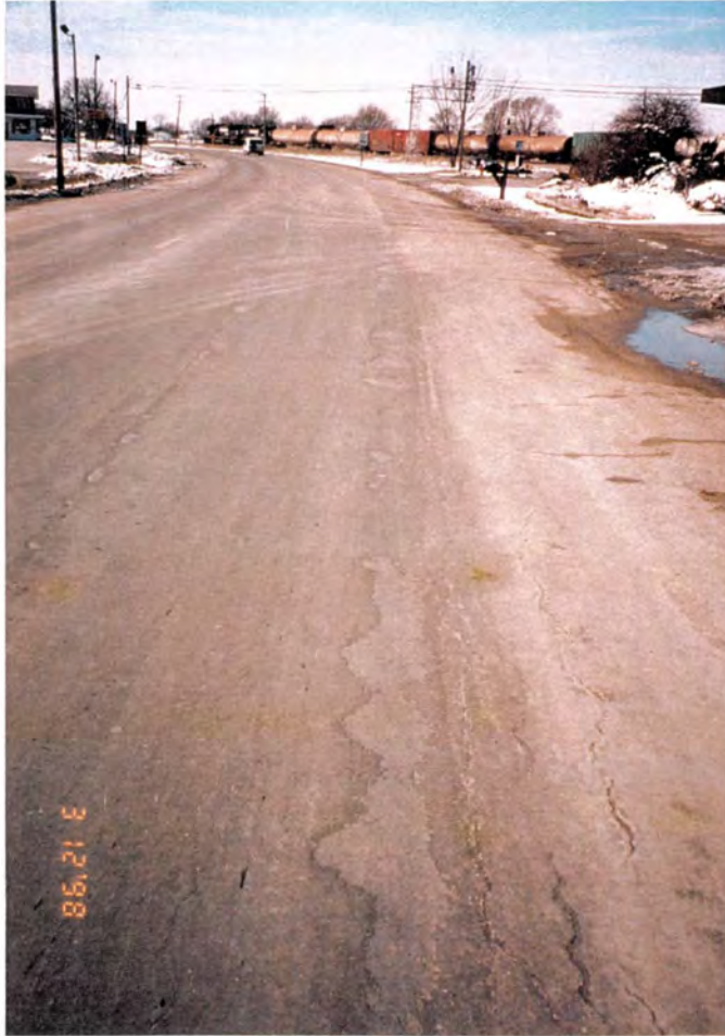
Photo #5: Loss of seal in wheelpath, near Route 24. March 12, 1998; District 2, Randolph County Route JJ
