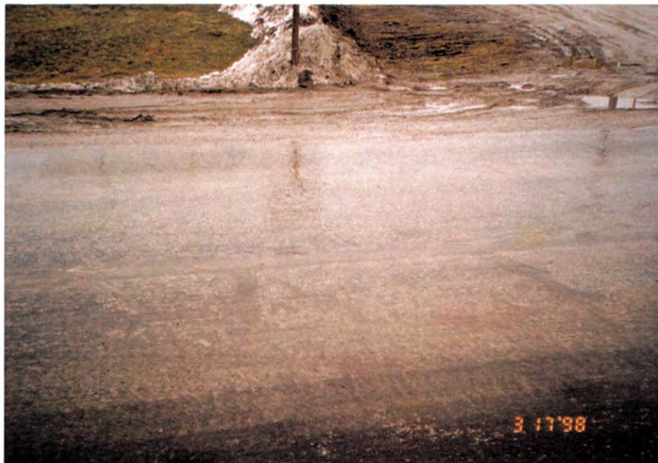
Photo #2: Wear and loss of seal on the surface. March 17, 1998; District 1, Andrew County Business Route 71
