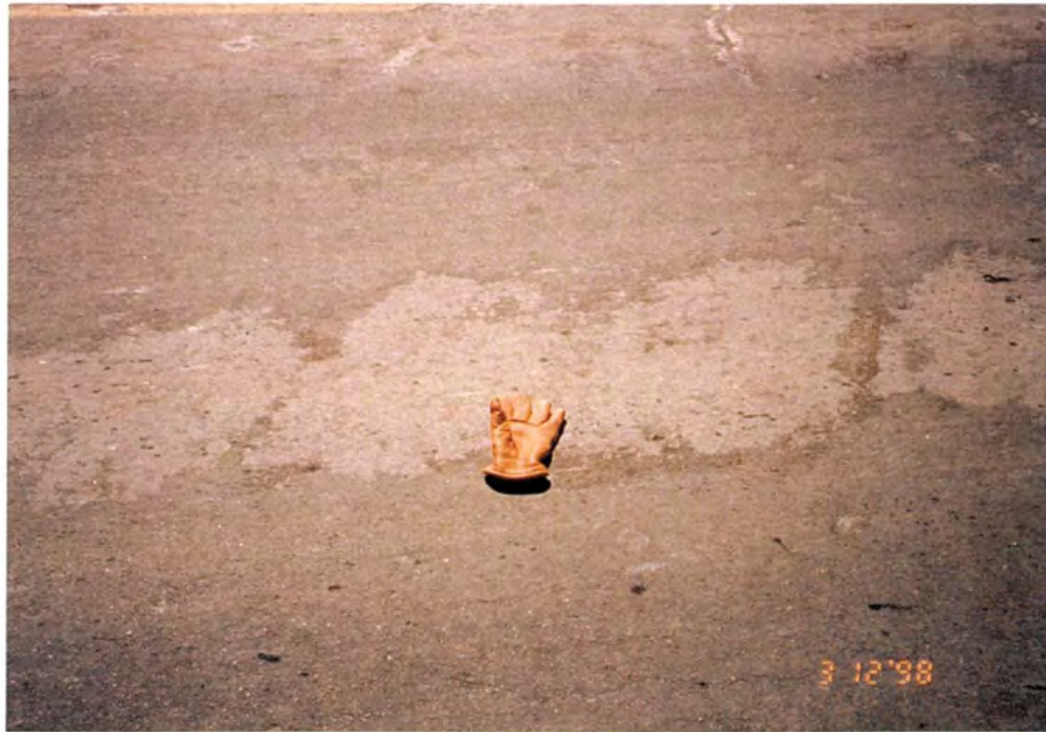
Photo #1: Loss of seal between the wheelpaths. A glove is shown for size reference. March 12, 1998; District 2, Randolph County Route JJ
