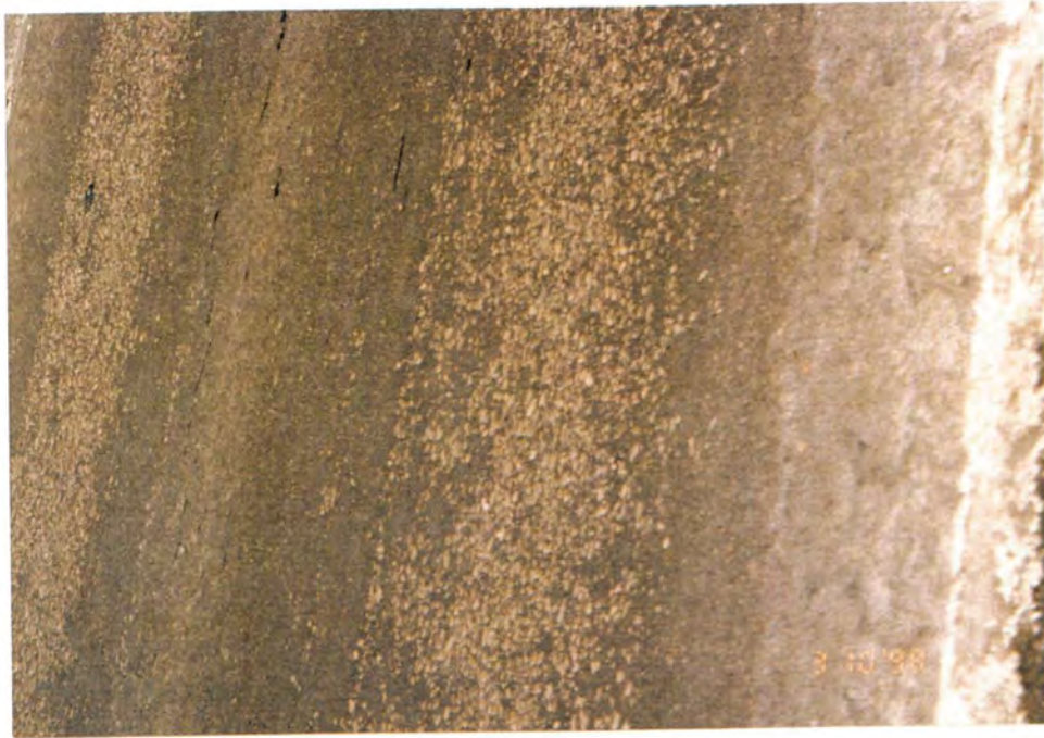
Photo #4: Two squares approximately 2' x 1.5' that has no seal. Several such areas were noticed on the south end of the project. March 10, 1998; District 6, St. Louis County Route 67 (Lindbergh Boulevard)
