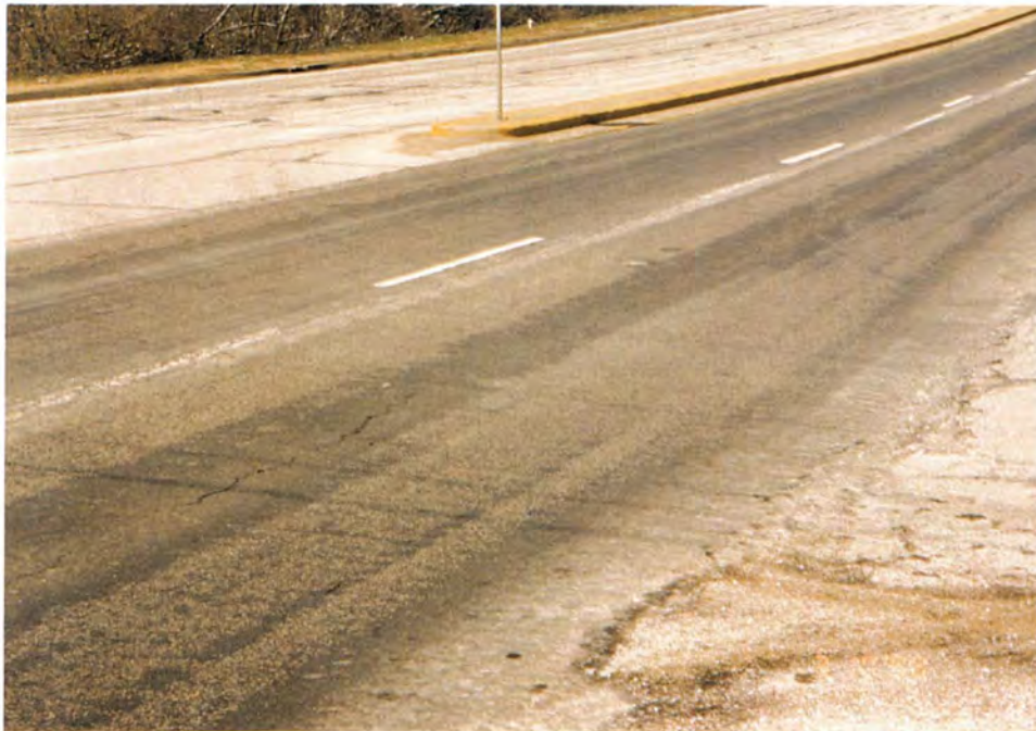
Photo #2: A close-up of the wheelpaths in this location. March 10, 1998; District 6, St. Louis County Route 67 (Lindbergh Boulevard)
