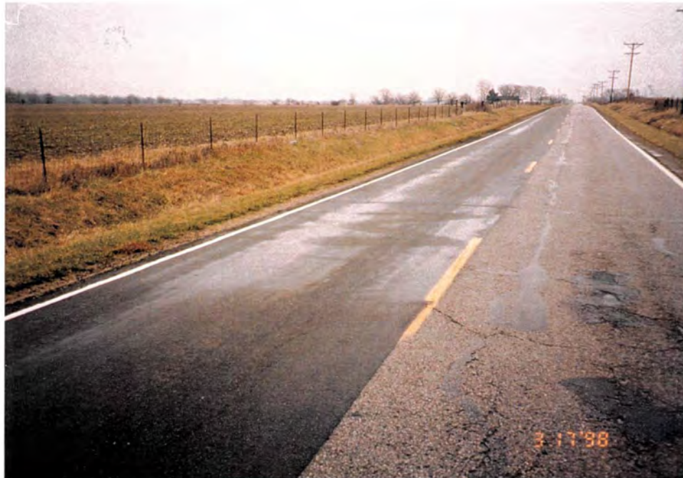
Photo #2: The lane on the left has been sealed; the one on the right has not. The seal appears to make a distinct difference in the quality of the driving surface. March 17, 1998; District 4, Henry County Route 52
