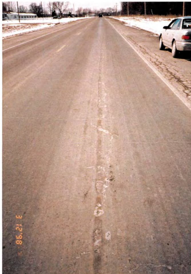
Photo #3: A series of small spalls in the seal. March 12, 1998; District 2, Randolph County Route JJ
