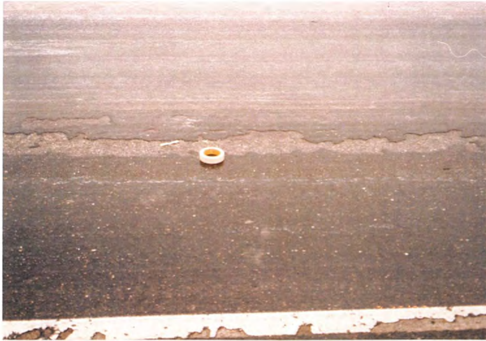
Photo #5: Loss of sealant on the driving surface. The roll of masking tape can be seen for size reference. March 16, 1998; District 2, Chariton County Route 24
