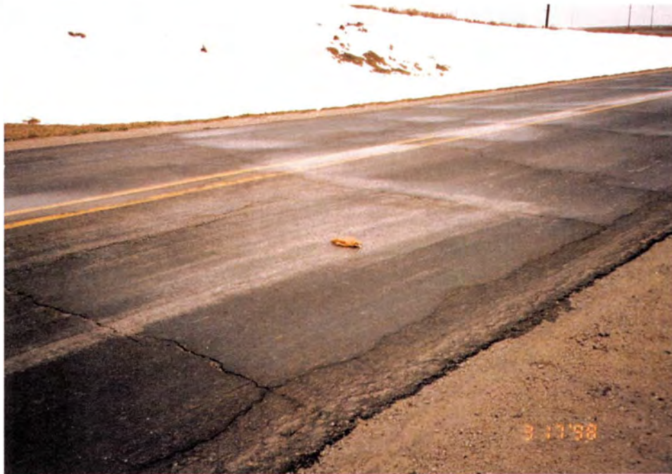
Photo #1: A scrape in the surface most likely due to a snowplow. March 17, 1998; District 1, Buchanan County Route JJ
