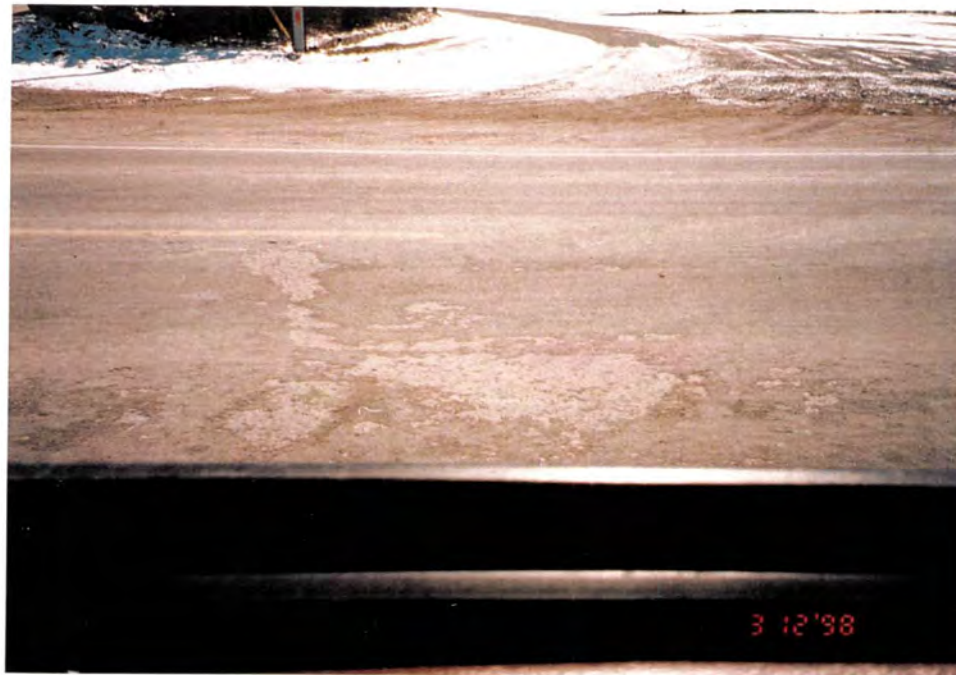
Photo #2: Loss of seal throughout the width of the lane. March 12, 1998; District 2, Randolph County Route JJ
