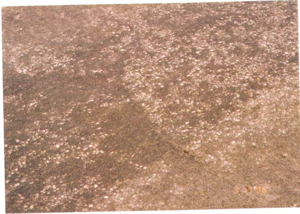
Photo #3: A close-up view of the surface showing wear and loss of seal. March 17, 1998; District 1, Andrew County Business Route 71
