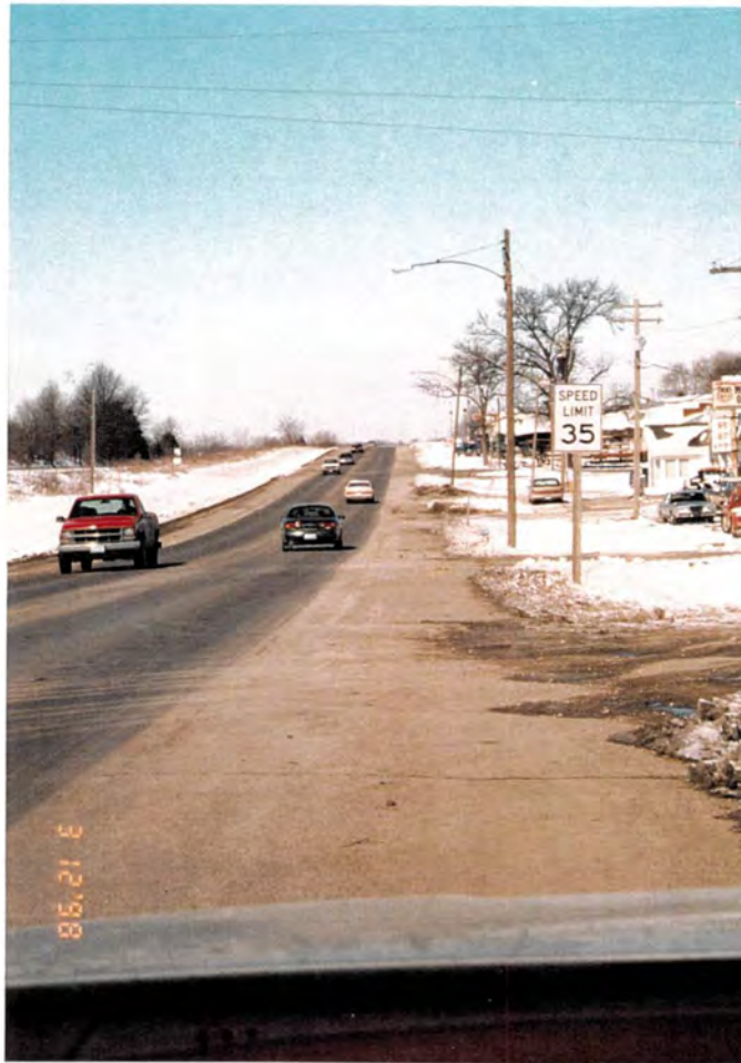
Photo #7: Another view of the surface. This seal is easily identified in this location due to its very black color. March 12, 1998; District 3, Audrain County Route 22
