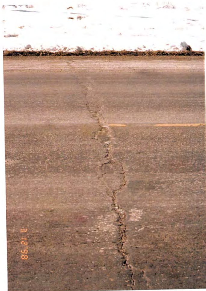
Photo #6: The sealant in a large pavement crack. March 12, 1998; District 3, Audrain County Route 22
