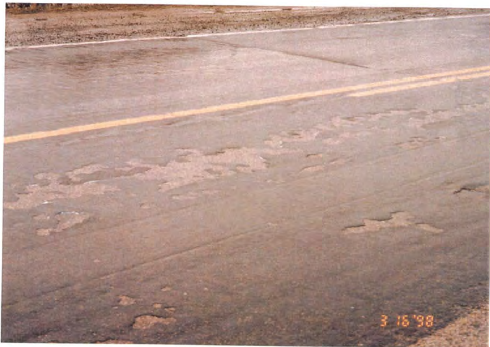
Photo #6: A close-up view of Photo #5. March 16, 1998; District 4, Lafayette County Route 24
