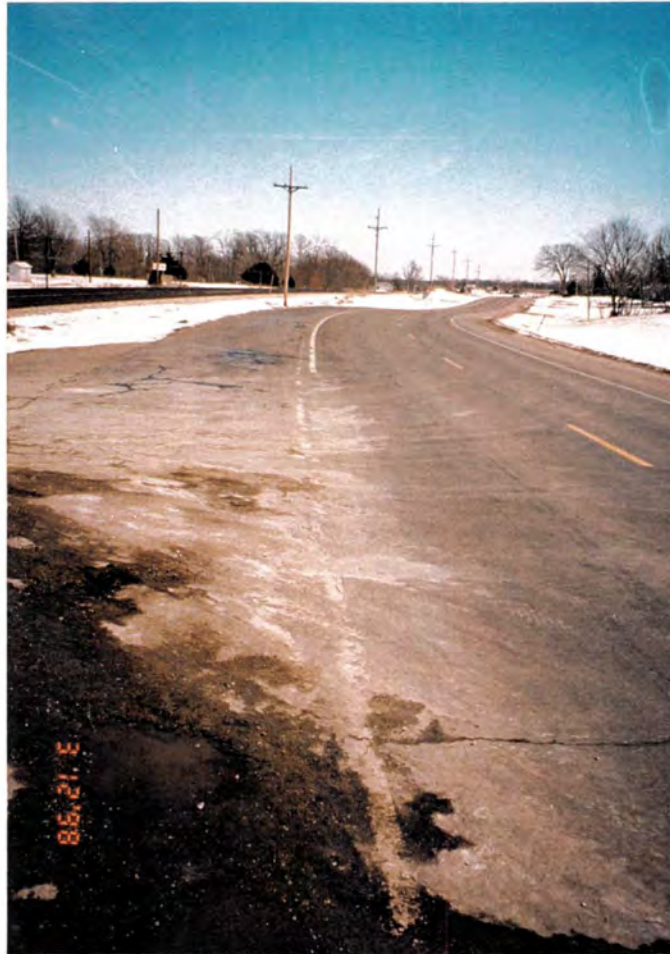
Photo #4: Loss of seal due to turning movements on a side road. March 12, 1998, District 2, Randolph County Route JJ
