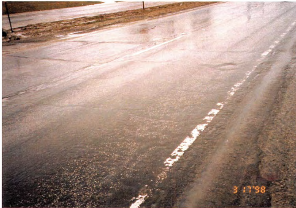
Photo #5: A second view of Photo #4 showing the difference in wear between the seal using sand as aggregate and wet bottom boiler slag as aggregate. March 17, 1998; District 1, Andrew County Business Route 71
