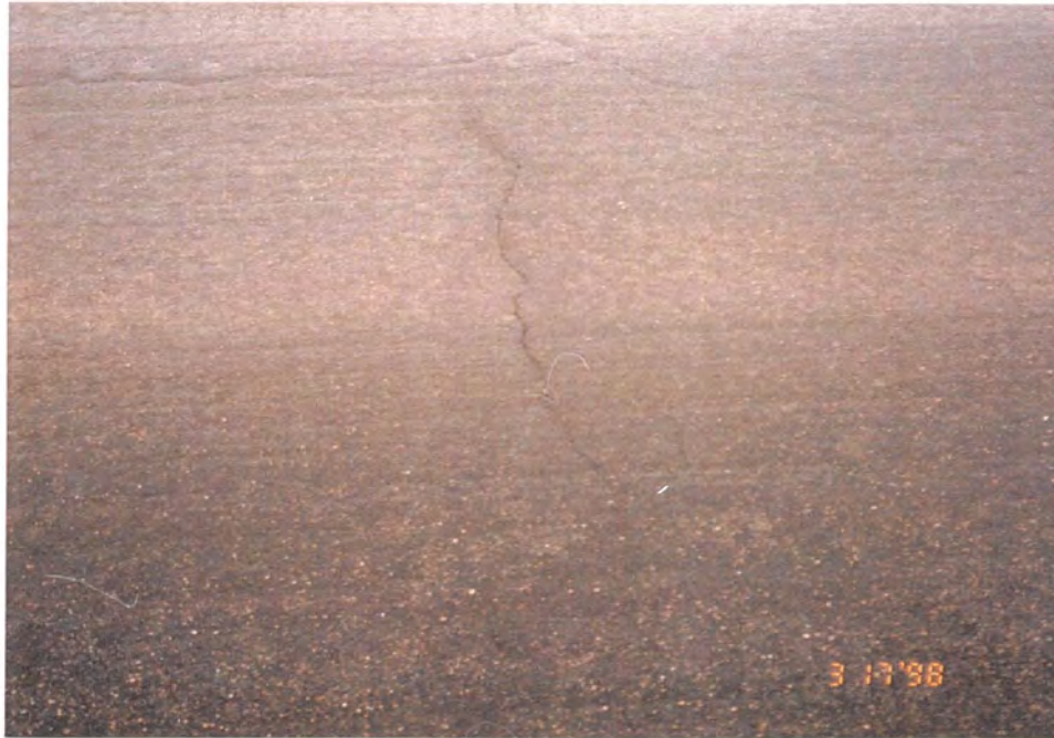
Photo #5: A view of a crack and the texture of the surface. March 17, 1998; District 1, Buchanan County Route JJ
