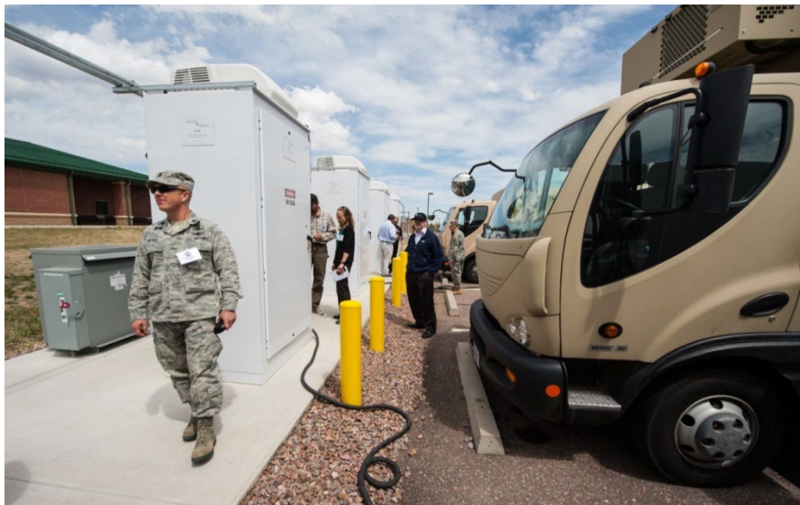
Bi-directional, fast-charging electric vehicle stations are capable of supplying power back to the Ft. Carson Army Base microgrid to help address demand or enhance overall power quality. (Photo by Dennis Schroeder /DOE-NREL)
