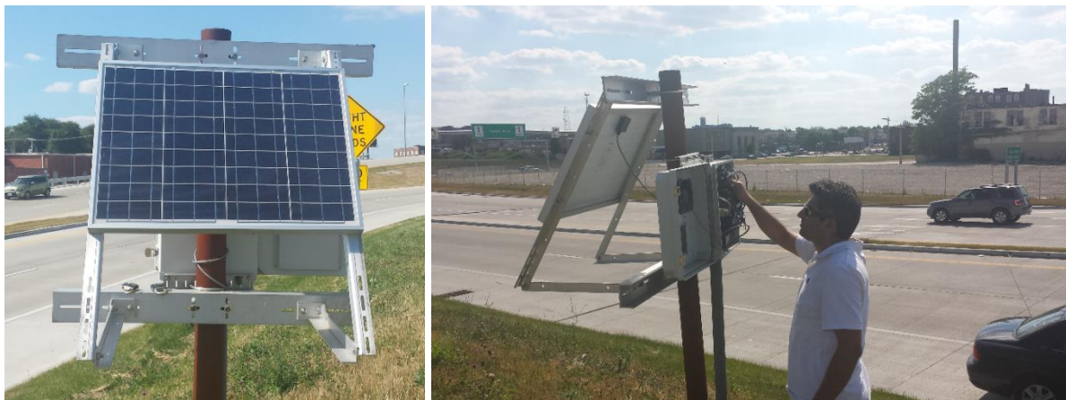
Figure 5-21. Solar powered data acquisition system and monthly data collection
