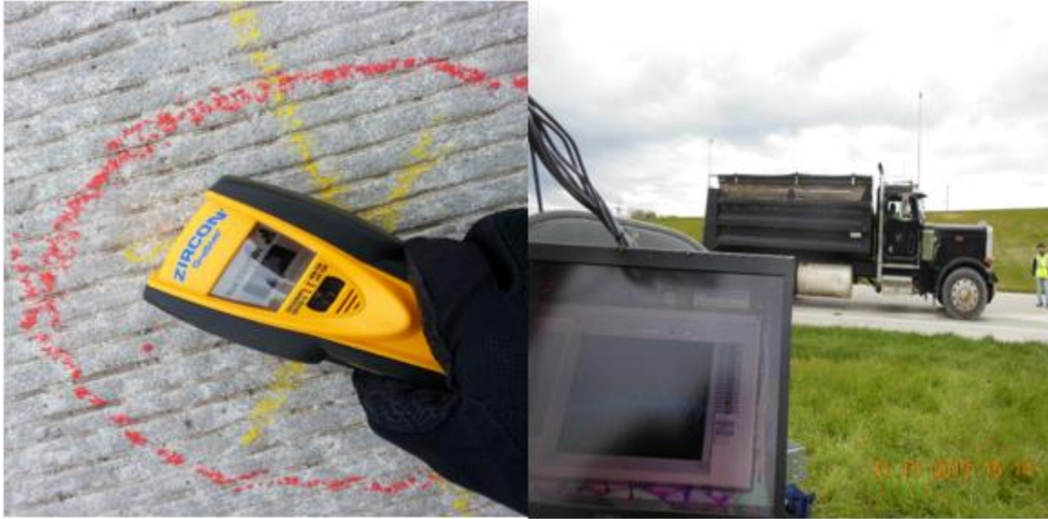
Figure 6-2. Deep metal scanner used for detecting sensor baskets (left) and simultaneous monitoring deformation to ensure exact location of sensors (right)
