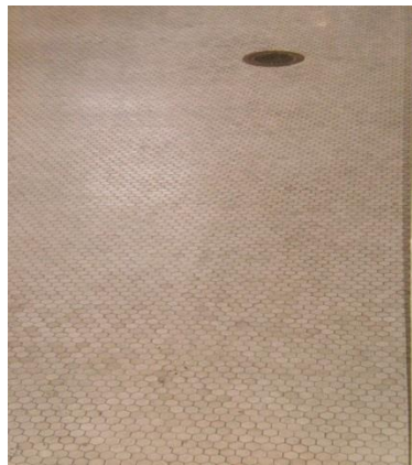
Figure 19. Lakeshores RCF Octogonal tiles in Operating Room Floor
