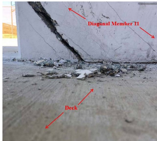
Figure 1-4 Cracking two before bridge collapse [2]
