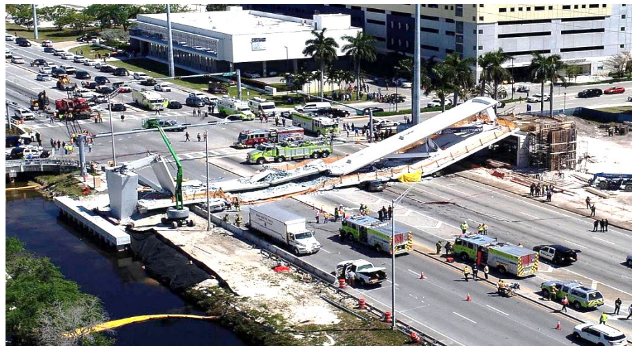
Figure 1-2 Full collapse of the main bridge segment [1]
