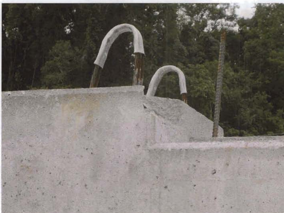
Figure 5.4 Breakout of Concrete at Lifting Loop
