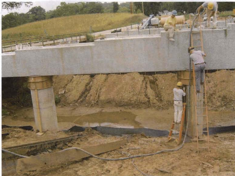
Figure 6.5 Grout Leakage and Sealing Leaks
