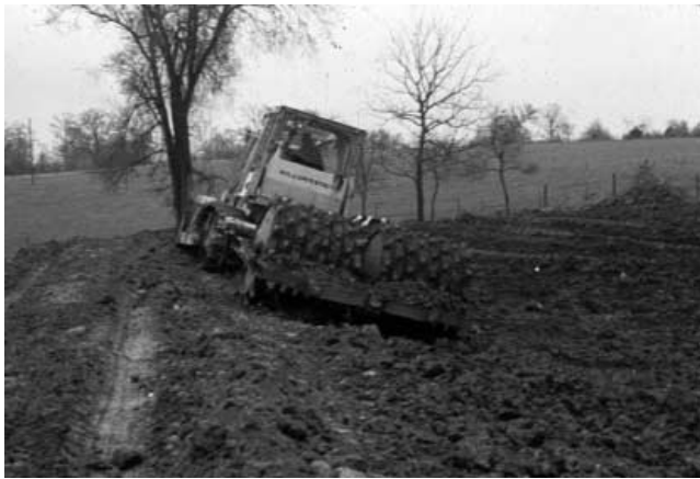
Figure 2. A sheep's foot roller is commonly used to compact the clay seal during construction of a lagoon.
