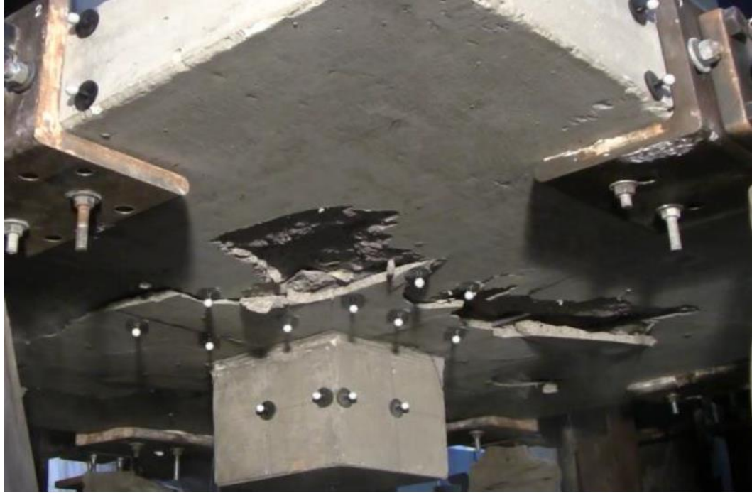
Figure 4.4.1.1 – Underside of 0.64% static test at punching failure of testing
