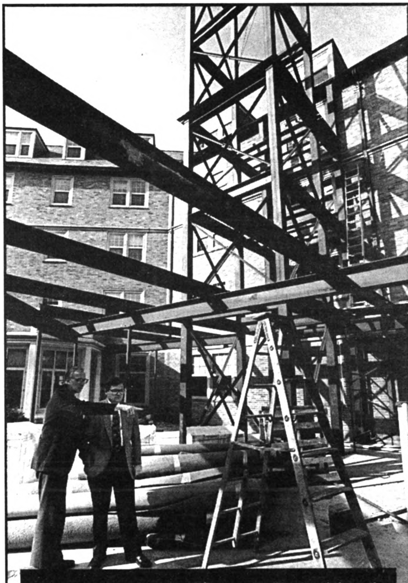
Campus Dining Services Director Jim Korner, left, and Roger Fisher, director of Residential Life, look over construction progress at Johnston Hall. An elevator and new dining facilities are the most visible changes at the hall.
