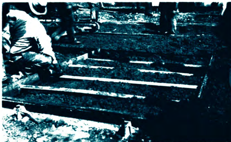
First batch spread and separators set preparatory to dumping second batch of concrete.
