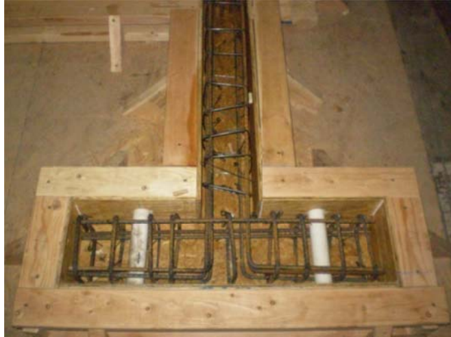
Figure 3.5.14: PCP pipe in pedestals
