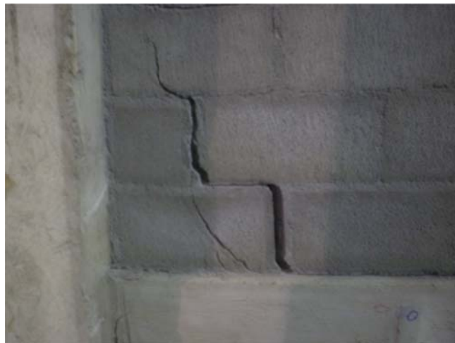
Figure 4.3.15: Initial crack near the center column
