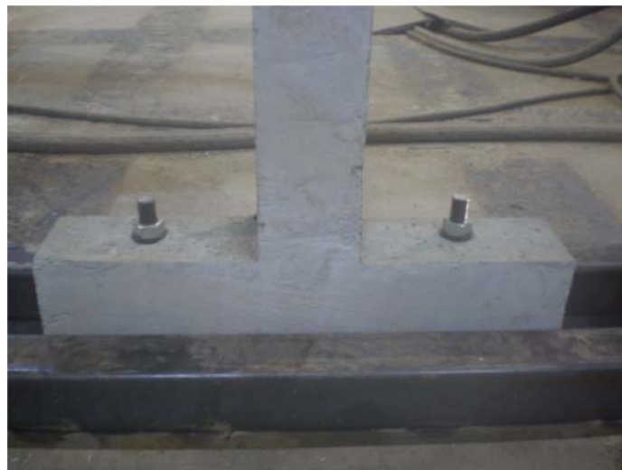
Figure 3.6.9: Pedestal anchored to the floor
