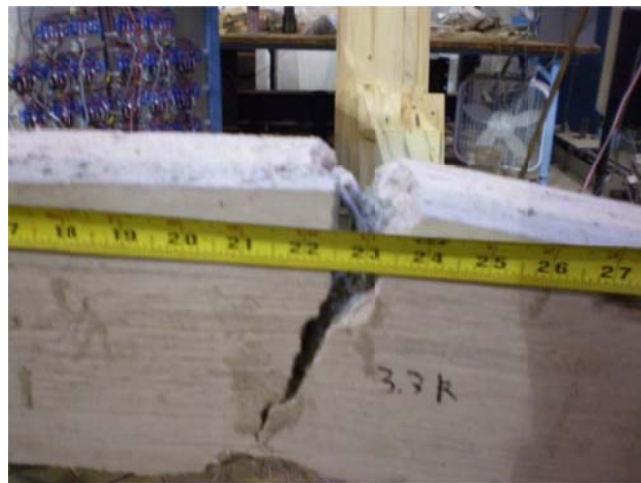
Figure 4.1.6: Crack at end of negative reinforcement
