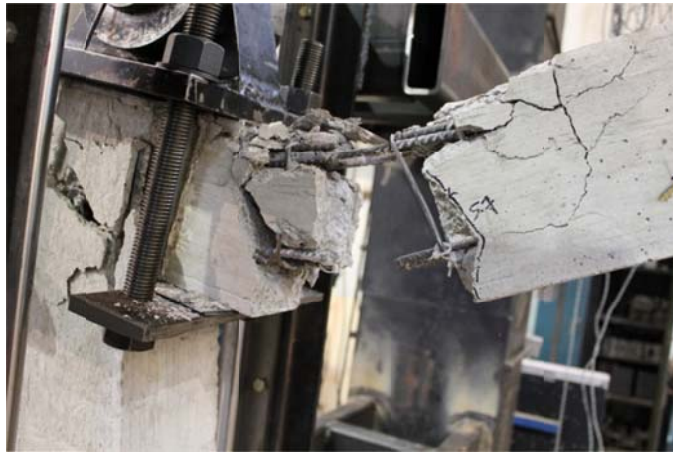
Figure 4.2.12: Bars fracturing near center column
