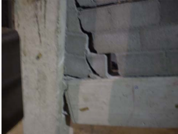
Figure 4.3.16: Crack propagates through beam and forms a hinge
