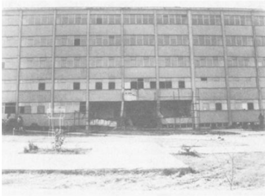
Figure 2.2.2: Office building damaged by system boiler explosion (Sucuoglu et al., 1994)
