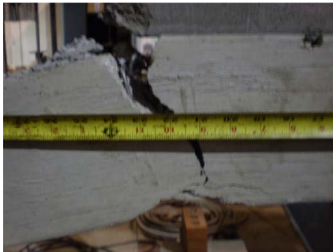
Figure 4.3.13: Crack formed where negative moment bars end
