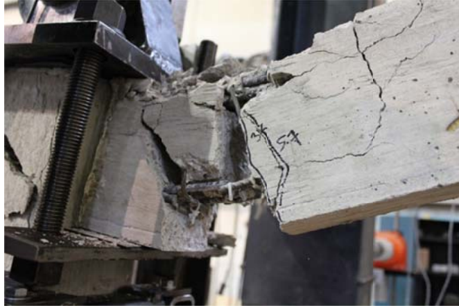
Figure 4.2.11: Hinge forming near center column
