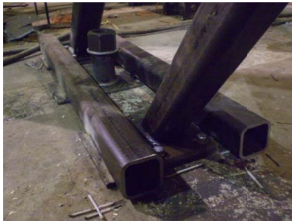
Figure 3.6.5: Reaction frame bolted into the structural floor
