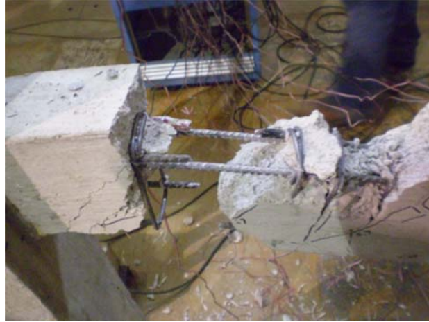
Figure 4.2.9: Failure of beam
