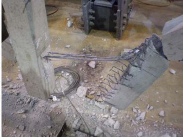
Figure 4.1.10: Longitudinal bars breaking out of the stirrups
