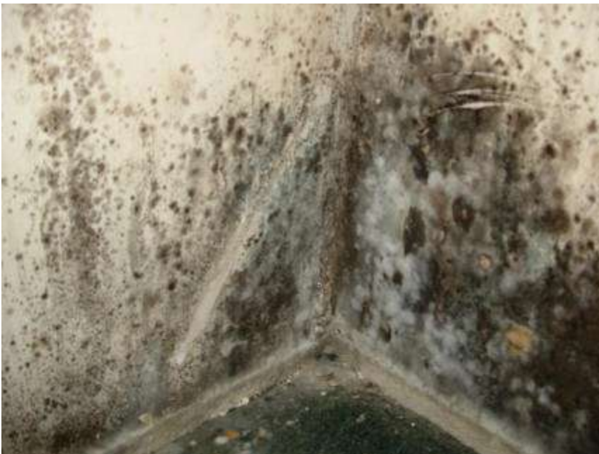
Figure 2.1 Black molds on wall
