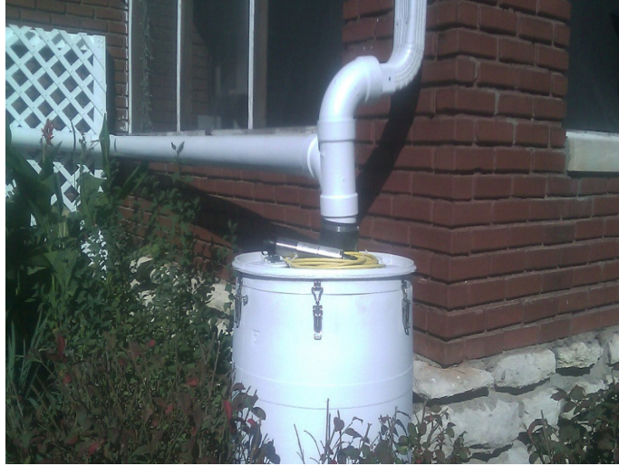
Figure 7.1 Rain garden inlet orifice-controlled flow monitoring device in barrel casing at the southwest corner of the residence.
