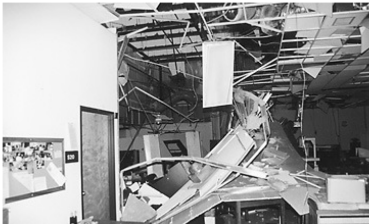
Damage to the microfilm lab in the Records Management/UM Press Building
