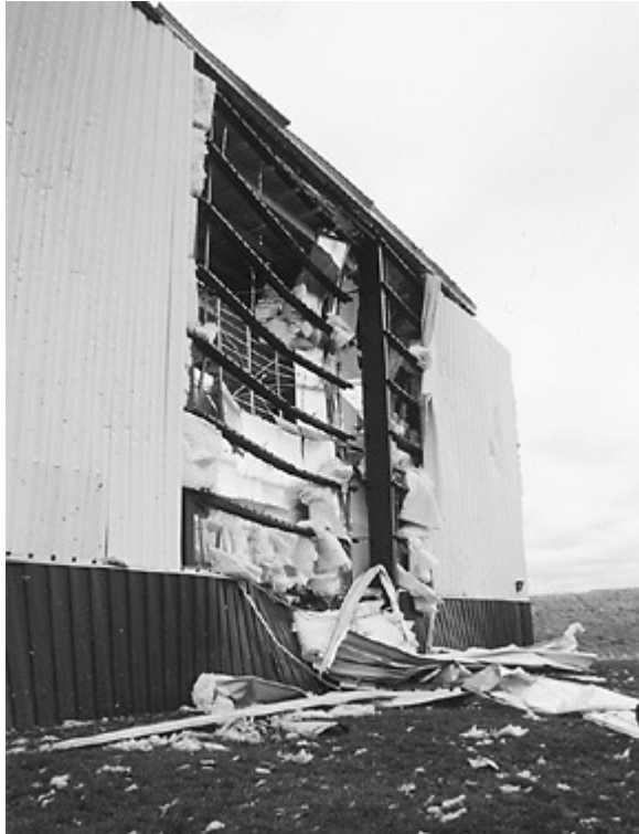
Damage to the UM Library Depository Building
