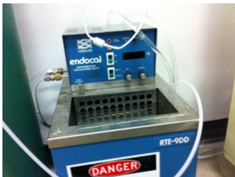
Figure 4.6 The Neslab chiller used to cool the M2 oil diffusion pump.
