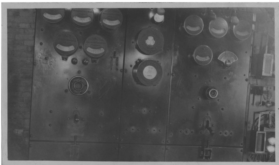
THE SWITCH BOARD.
