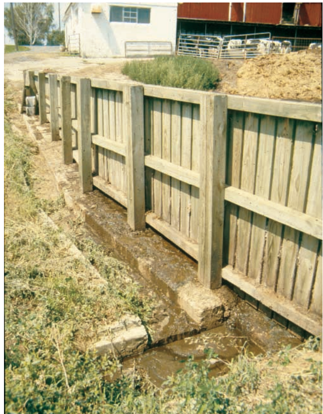
Figure 2. A concrete trough collects runoff that drains through this picket dam.
