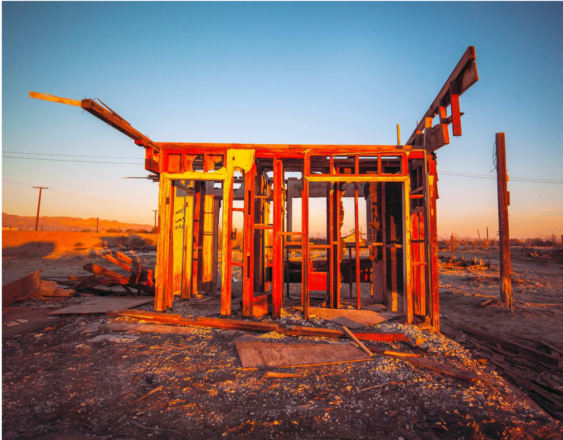
Abandoned building in the flooded part of Bombay Beach
