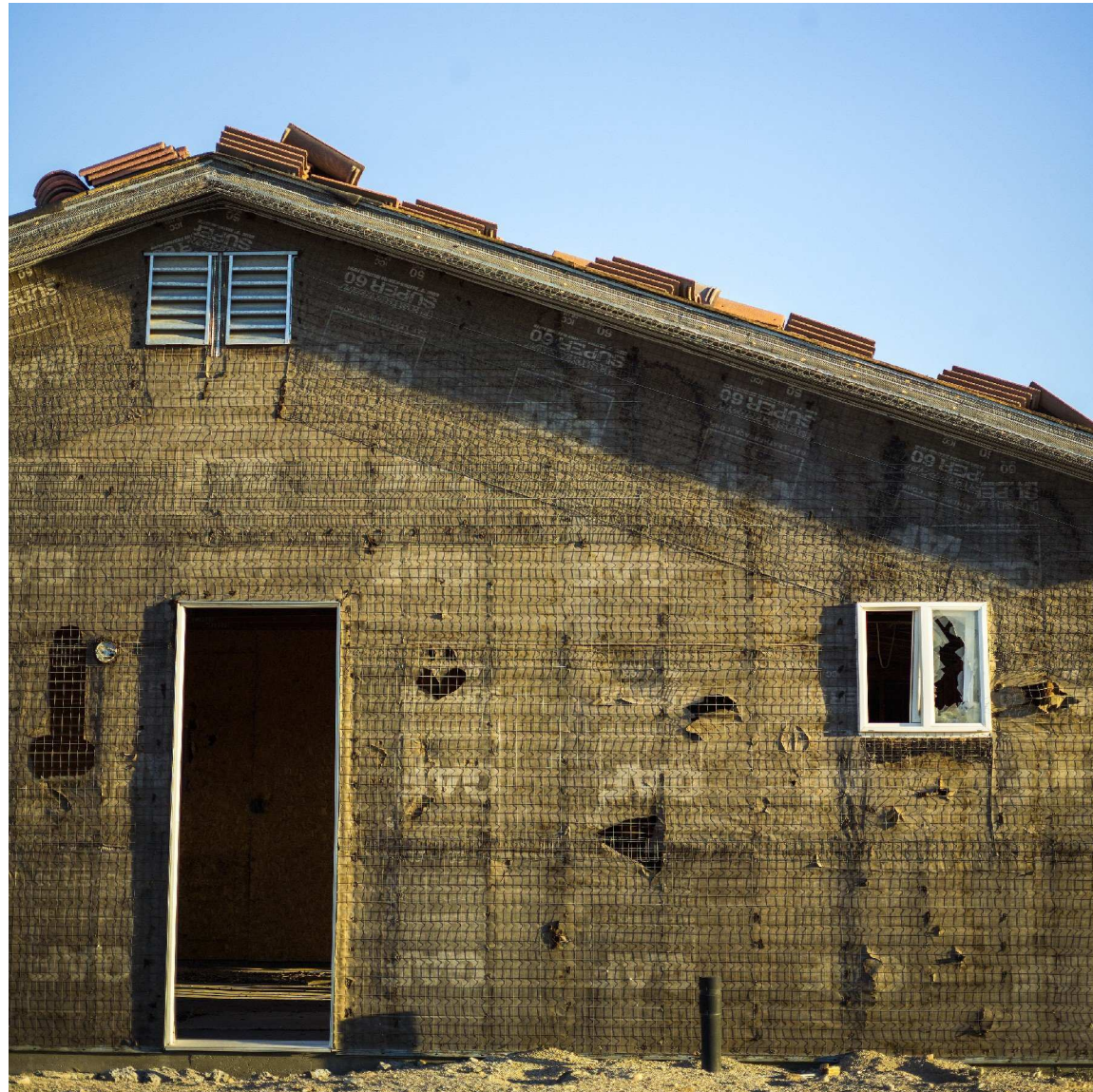
Home abandoned while under construction in Salton City. There was a spurt of new building in Salton City, which abruptly ended in October 2008 after the Great Panic and the California housing market bubble burst. This house and others in the area are half-built, with insulation, windows, plumbing, and electrical already installed.
