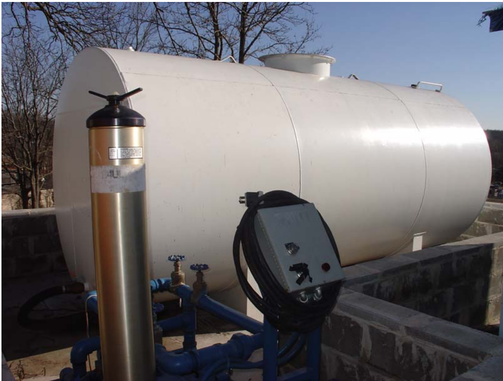
Figure 2.5. Secondary oil storage tank
