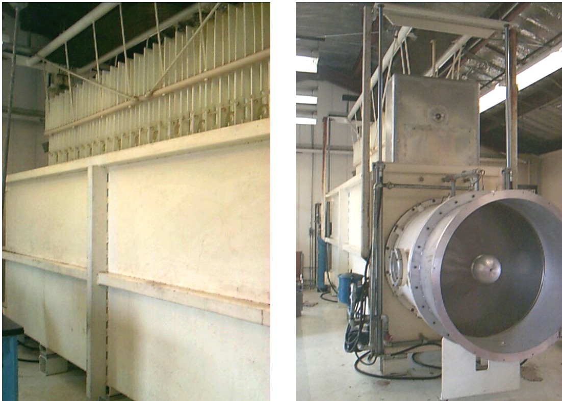
Figure 2.4. Indoor oil containment tank with capacitors in raised position
