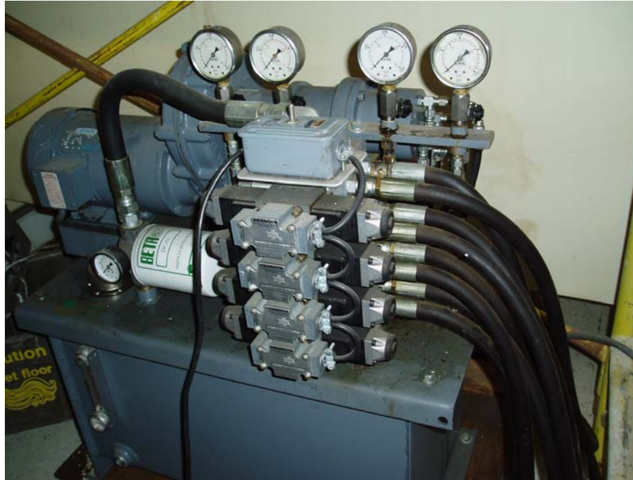
Figure 2.3. Hydraulic pumping system
