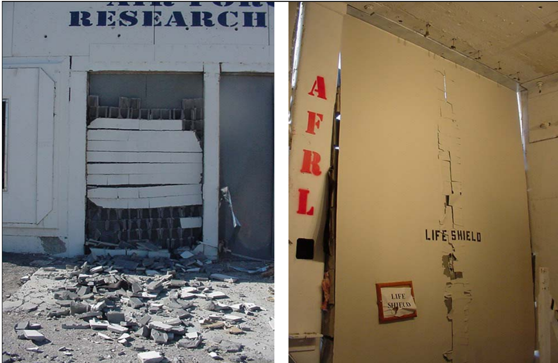
Figure 5.11 – Outside and Inside of Wall after Explosion
