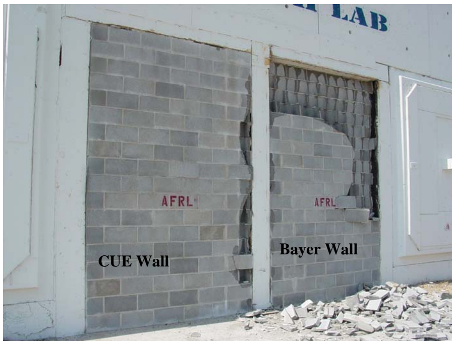
Figure 5.19 – Outside of CMU Wall after Explosion
