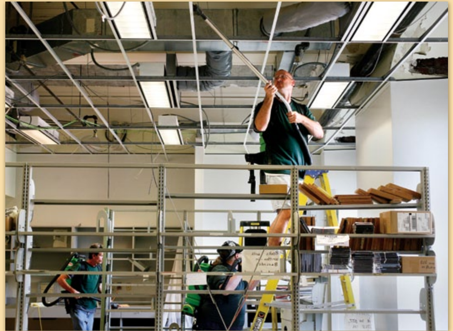
Workers clean the ceiling in the circulation area. Photo by Nicholas Benner.
