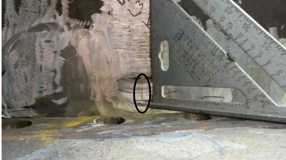
Figure 1-2: Vertical crack located in the SMB arch tie butt weld.
