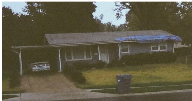
Figure 60. Home with tarp on roof.
