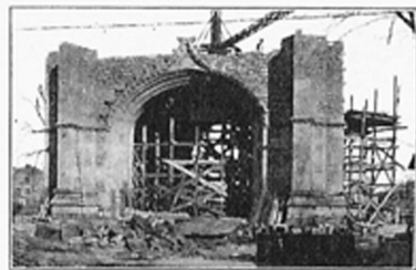
The open spring weather has permitted rapid progress on the construction of the Memorial Tower. Several feet of stone has been added since this photograph was taken.
