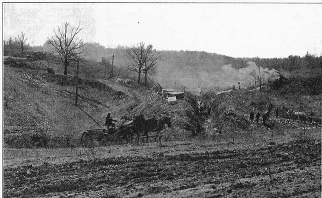
Work on the stadium is going on in earnest. Three shifts of men are employed. This view is from the south end of the ravine looking toward the golf course.
