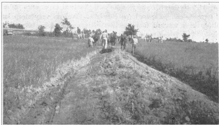
Fig. 12.—A terrace being constructed with a small blade pulled by a 4-mule team. Warren County.
