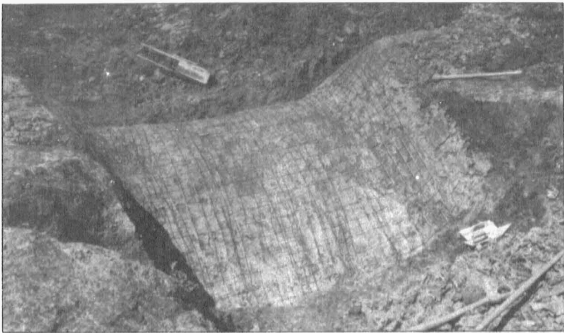
Fig. 2.—Downstream side of shaped earth form. This earth form at the end of a terrace outlet is ready to be covered with concrete and will carry water from a terraced field in Scotland County. Notice the heavy hog wire which will be in the middle of the 4-inch layer of concrete.
