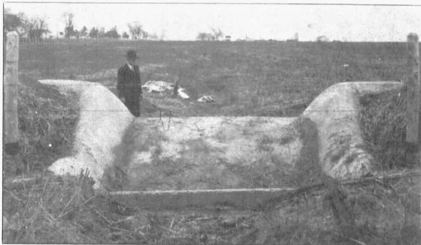
Fig. 8.—The downstream side of the same structure as in Figures 6 and 7, with baffle and stilling basin shown. Notice the rolled edges of the structure and the flat apron on which the water will fall after striking the baffle velocity check. This structure will carry water from approximately 40 acres of terraced land coming from a wide grassed outlet to be constructed along the fence seen on the left and not from out in the field where the old gully was located.
