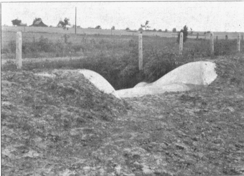
Fig. 7.—The same structure as shown in Figure 6 after backfill is properly made. Note the wings are completely covered and the earth is puddled in to the approximate level of the notch.
