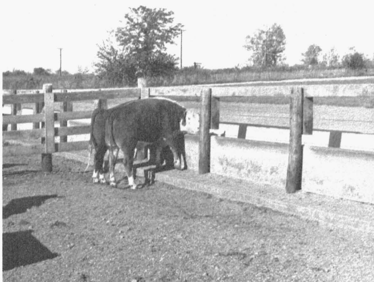
Erosion of fill from too narrow apron requires extra maintenance to correct this awkward situation (lot 6).
