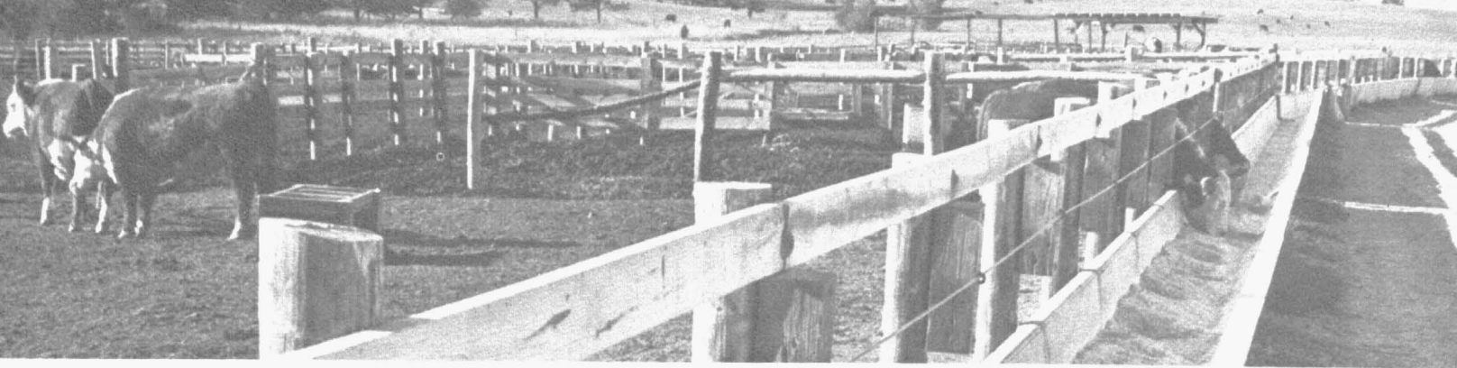
Precast concrete feed bunks were set in position with a wench truck.
