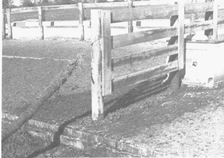
Spillage from waterers led to some erosion of fill adjacent to the concrete aprons.
