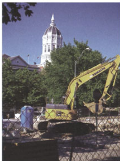
Publications file photo In this July view of Conley Avenue, construction workers replace the 1923 steam tunnels that provide heating to campus buildings and install chilled water lines that provide energy-efficient air conditioning. Conley reopened in mid-August in time for the students' arrival for fall semester.
