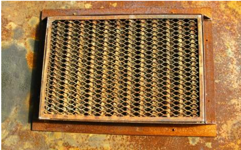
Figure 13. Ventilation System , detail, 2007.
