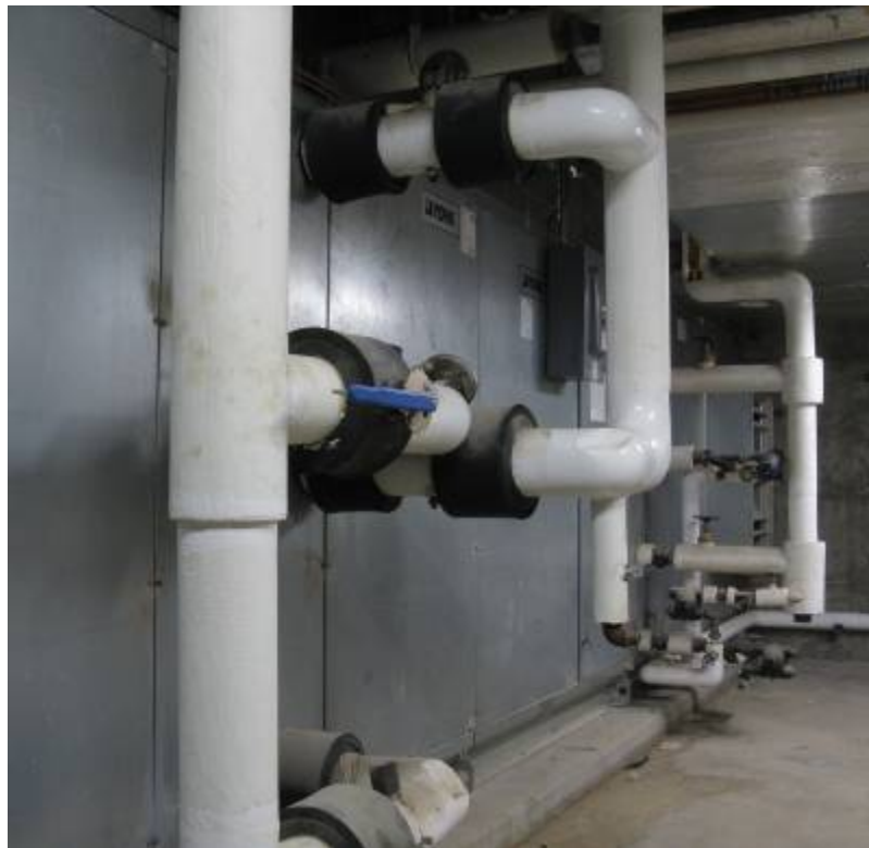
Figure 11. Photograph of an air handler.
