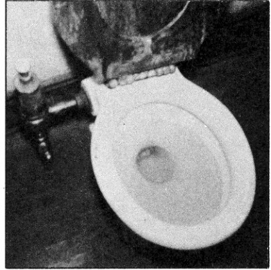
Fig. 32.—A side spud flushometer valve at a church with no vacuum breaker.
