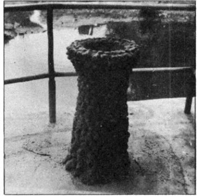
Fig. 59.—A fountain near an outdoor swimming pool. This supply also comes up through the waste line.
