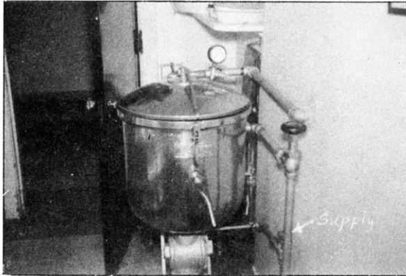
Fig. 28.—A bed pan washer at a hospital with submerged supply. These are always to be considered a definite hazard to the water supply when installed in a manner similar to that shown.
