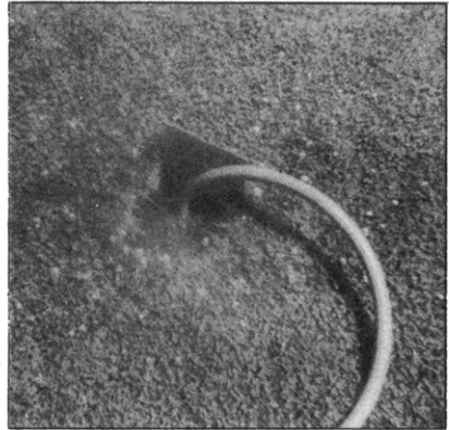
Fig. 79.—A yard hydrant that is filled with water around the leaking hose connection. The supply valve is entirely submerged in this contaminated water.
