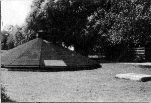
Fig. 11.—A view of one of the wells which supplies the reservoir. (Concrete block near right edge.) The reservoir is supplied by four four-inch wells in the bottom of the reservoir and one eight-inch well outside, each of which is 85 feet deep.
