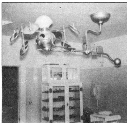
Fig. 27.—A view of the operating room displaying an expensive bank of lights by which to operate. Post-operative infections have occurred in numerous cases from such installations as shown in Fig. 26. This is the hospital, mentioned earlier, in which there is a plugged sewer line and water supply lines which are heavily encrusted.
