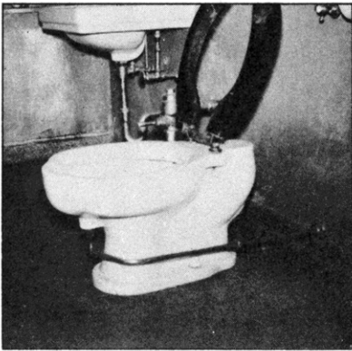
Fig. 33.—A flushometer valve at an infirmary with no vacuum breaker.
