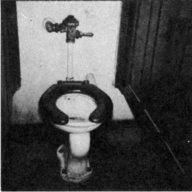
Fig. 31.—A flushometer valve at a school with no vacuum breaker.
