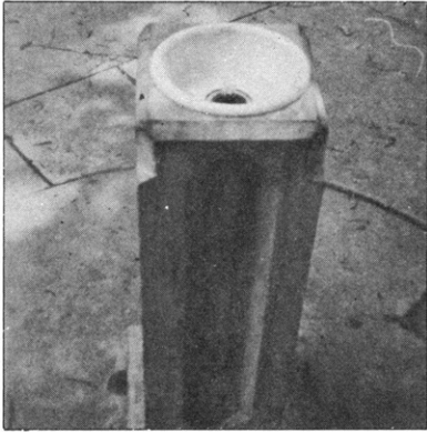
Fig. 58.—Outdoor fountain with inverted bubbler supply which emerges from the waste line and terminates below the overflow level of the fountain.
