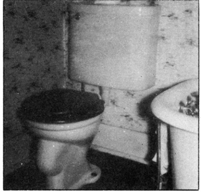
Fig. 36.—A water closet wall-supported, submerged valve supply. This is a common defect.
