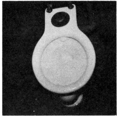
Fig. 34.—A side spud flushometer valve at a school with no vacuum breaker.
