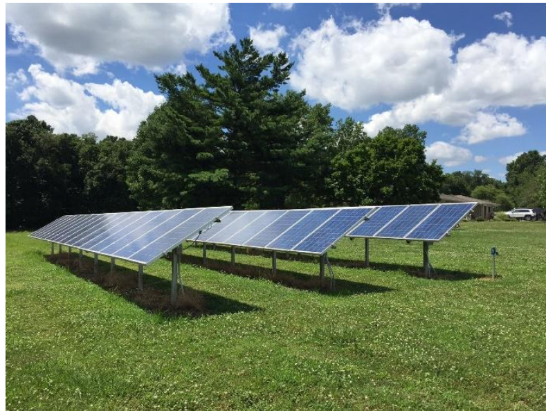
Image 6. The Surveyor's ground mounted PV array
