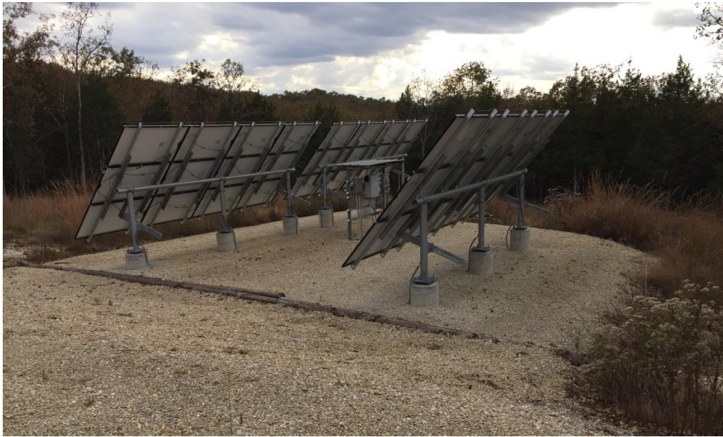
Image 15. The Engineer's PV array on an adjustable racking system
