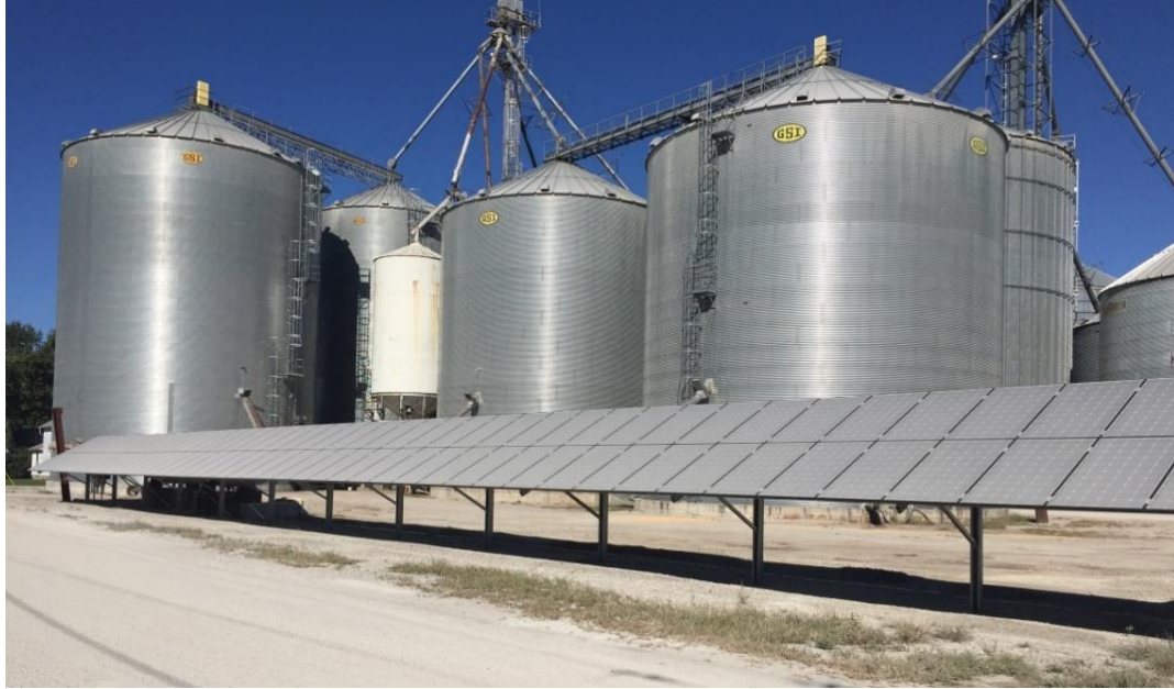
Image 21. Large ground mounted PV array at a grain elevator
