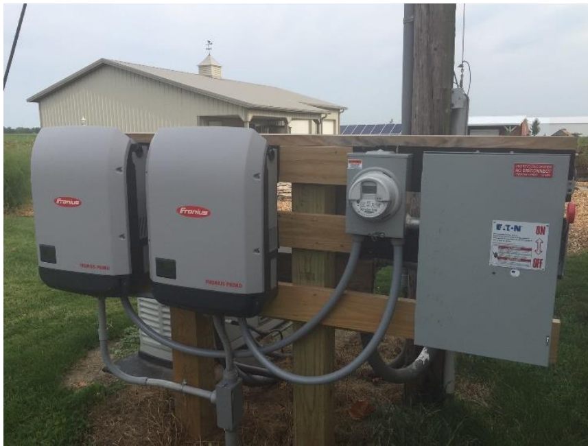
Image 18. Primary disconnect switch on breaker box, net meter, and micro inverters
