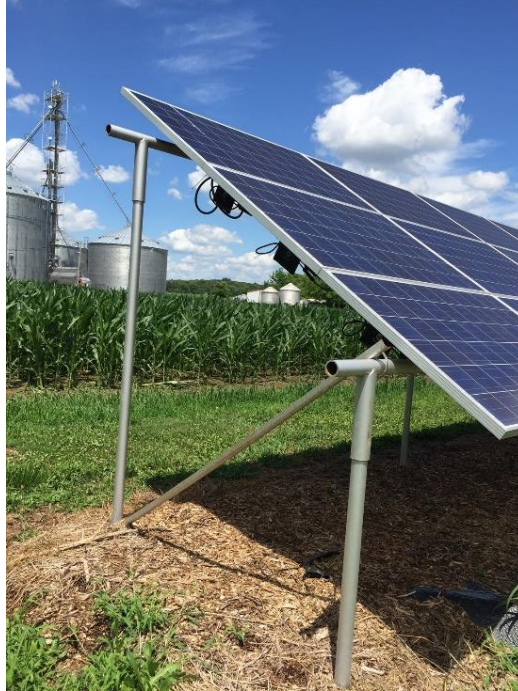
Image 7. The Surveyor's uncle's ground mounted PV array
