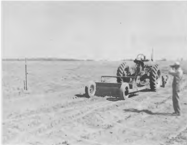
Fig. 13—Checking to determine if the terrace channel has been excavated to the proper depth.
