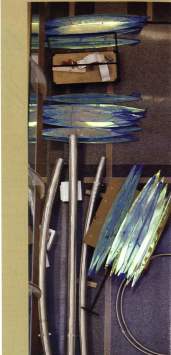
Building blocks of art are arrayed on the floor of the McQuinn Atrium. When complete, braided stainless steel cables suspend acrylic helixes and enlarged microscope slides of current research around a brushed aluminum spine of the Joy of Discovery .
