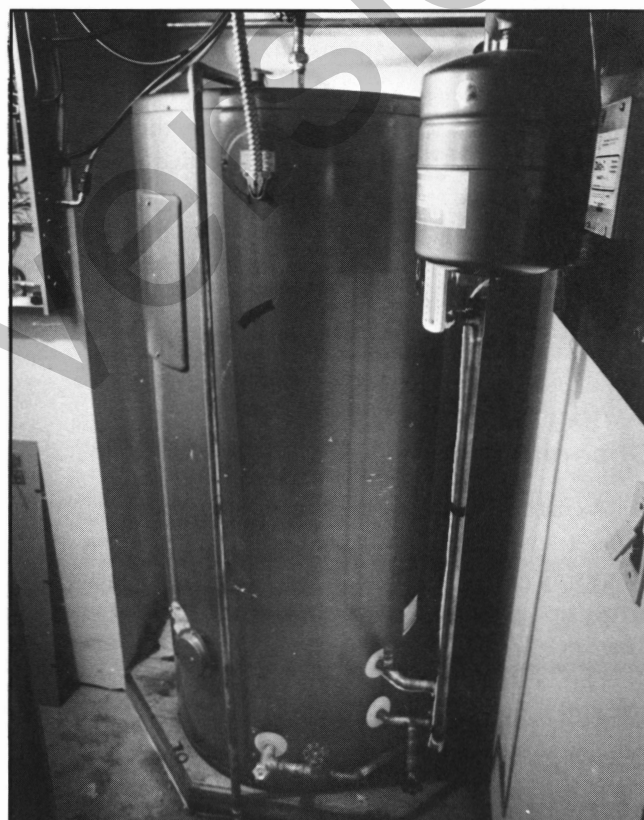
120 gallon storage tank weighs 1,500 pounds when full. Flexible conduit near top leads to single 4,500 watt back-up element.
