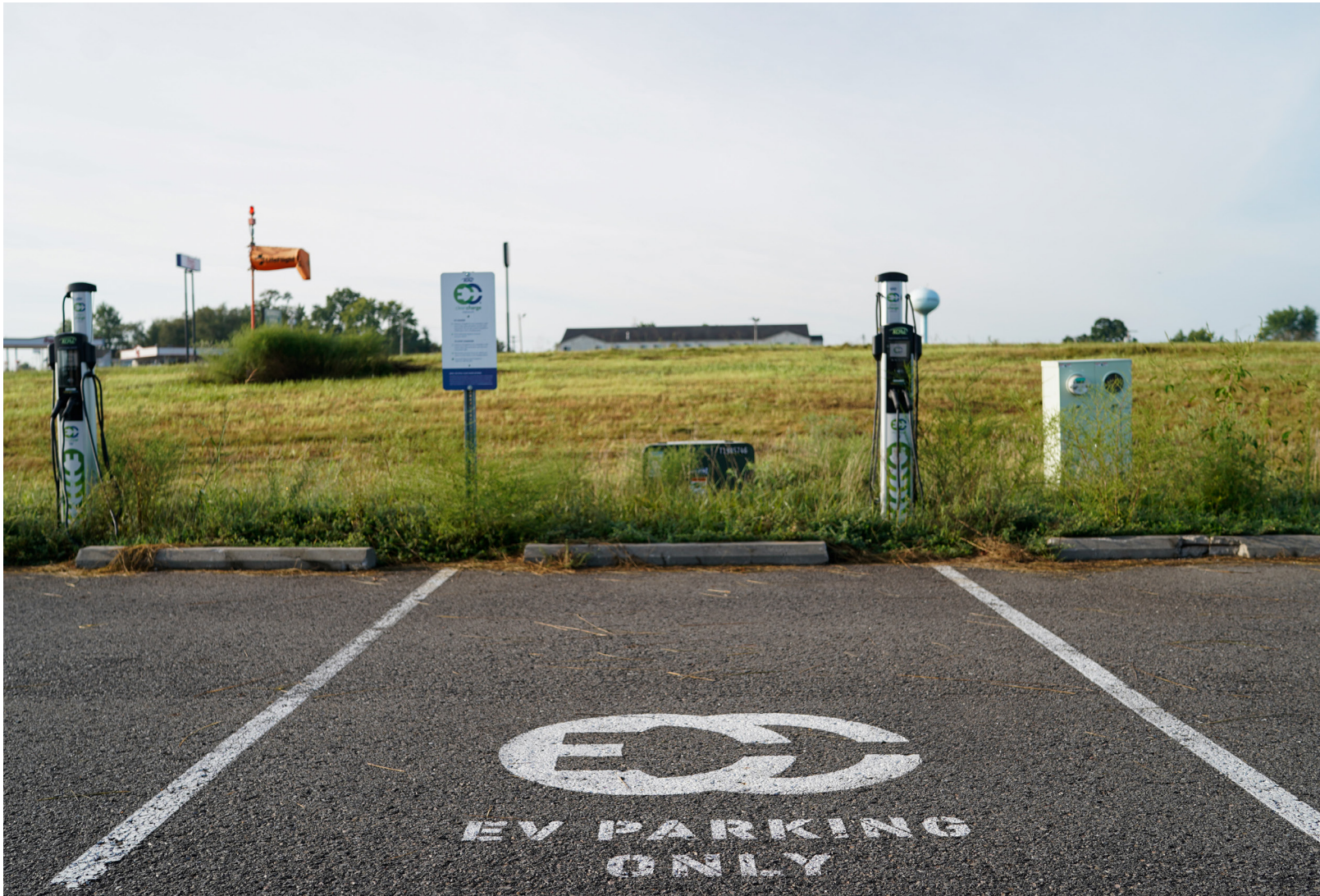
EV parking spot on the I-70 Community Hospital's parking lot.
