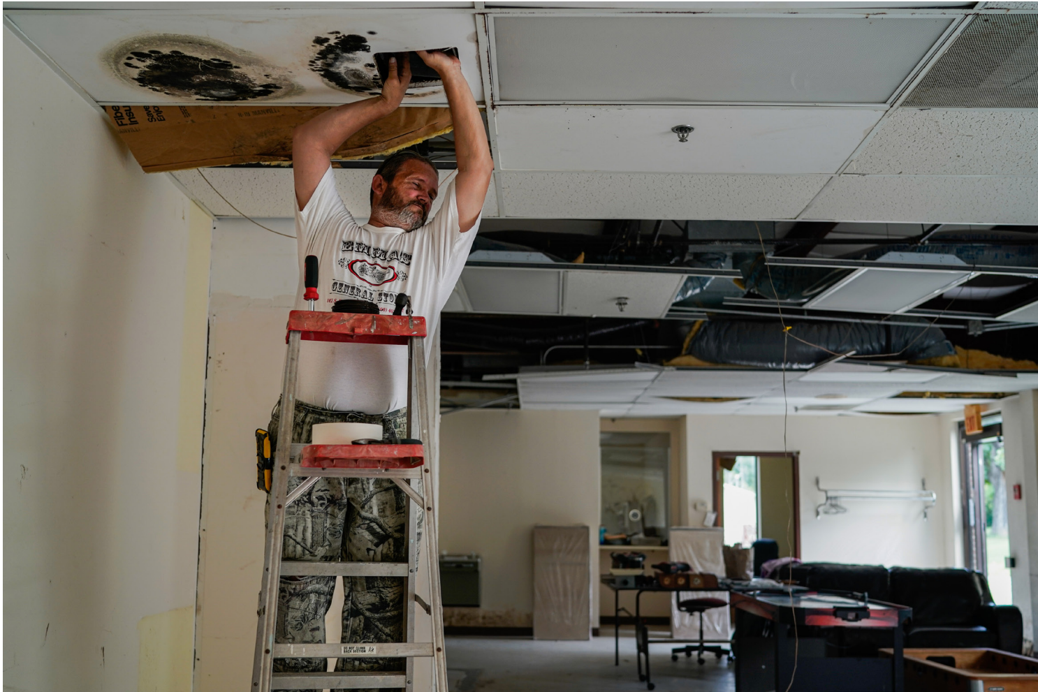
August 24, 2019 Kevin Browder volunteers to help in the old hospital. Joe Campbell leads the old hospital renovation project in town. A youth center will be put inside the building for kids in the community.
