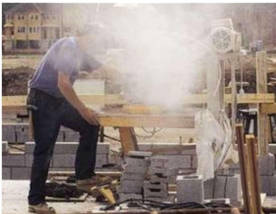
Figure 2: Fugitive dust blown into the air from a concrete saw. (Slate Health and Safety)
