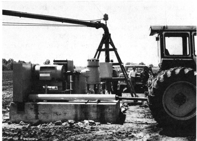
Figure 3. Mechanically started electric motor (Central Power Systems photograph).
