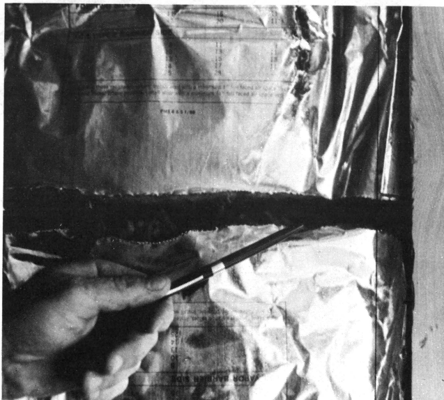
Figure 2. Poor workmanship during installation is a major problem with insulation in today's home. The poor fit shown here leaves an uninsulated area of the wall which the homeowner will probably never see, but which will add cost to every fuel bill.
