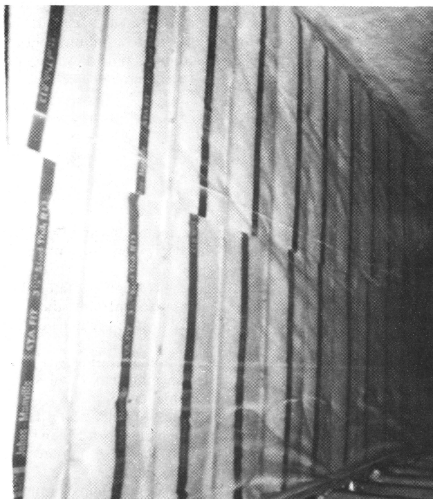
Figure 3. This well insulated exterior wall section contains 3½-inch-thick fiber glass batts. A clear polyethylene sheet has been placed over the batts to act as a vapor barrier. Clear polyethylene provides an excellent vapor barrier and has good transparency so carpenters or dry wall installers can see stud faces easily when they apply the interior wall covering. A one-inch thick expanded polystyrene sheathing board on the outside surface of the studs brings total R-value for wall insulation to 18.
