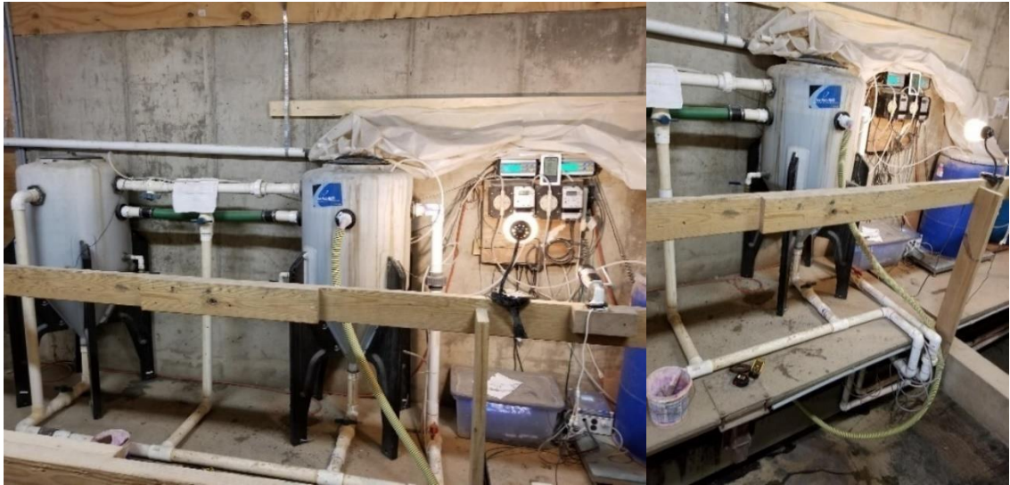
Figure 12. Recirculation line from acid tank to the trough, June 19.
