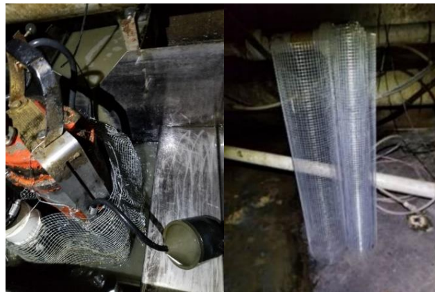
Figure 15. Foaming deactivated the float switch, led to continuous pumping and excessive foaming (July 19), and installation of a filter screen (removed later).
