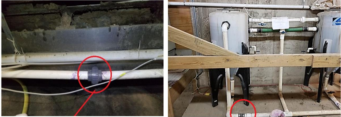
Figure 14. Self-aligning union and rubber couplings added to simply add an access to the system for cleaning.
