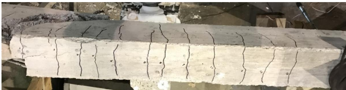
Figure 3-54. Locations of the measured cracks (B9-SL).
