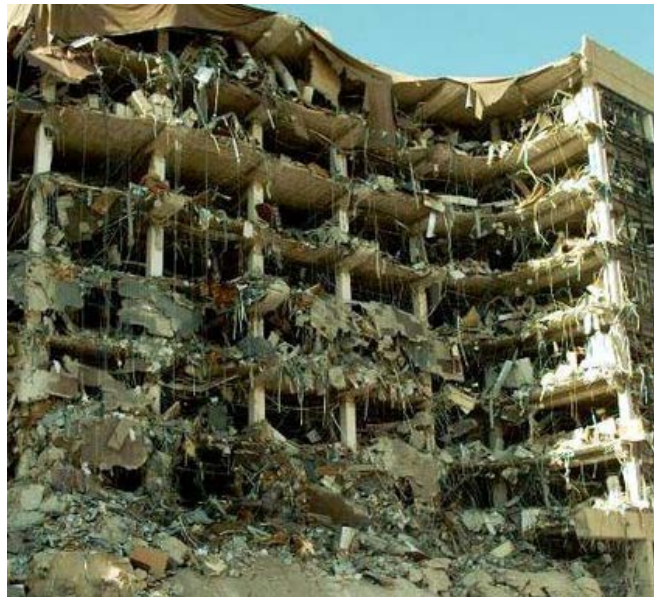
Figure 1: Bomb attack on Murrah Federal Building in Oklahoma, USA, 1995 (Hidallana-Gamage, Thambiratnam, & Perera, 2015).
