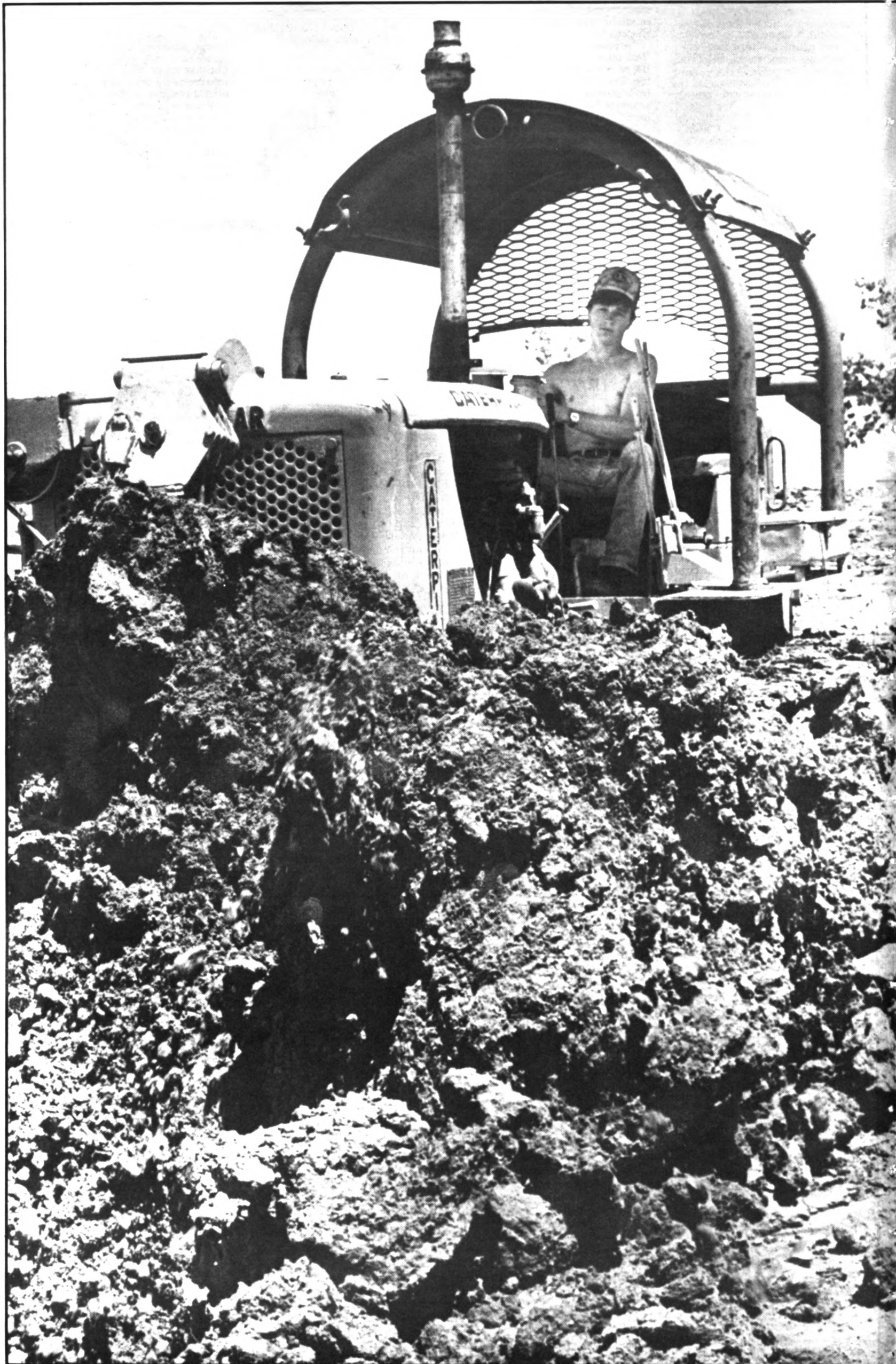
Student Eric Cowan works on the first phase of Stankowski Field redevelopment, which will result in a more durable turf, better drainage, two larger recreation fields and a jogging path.
