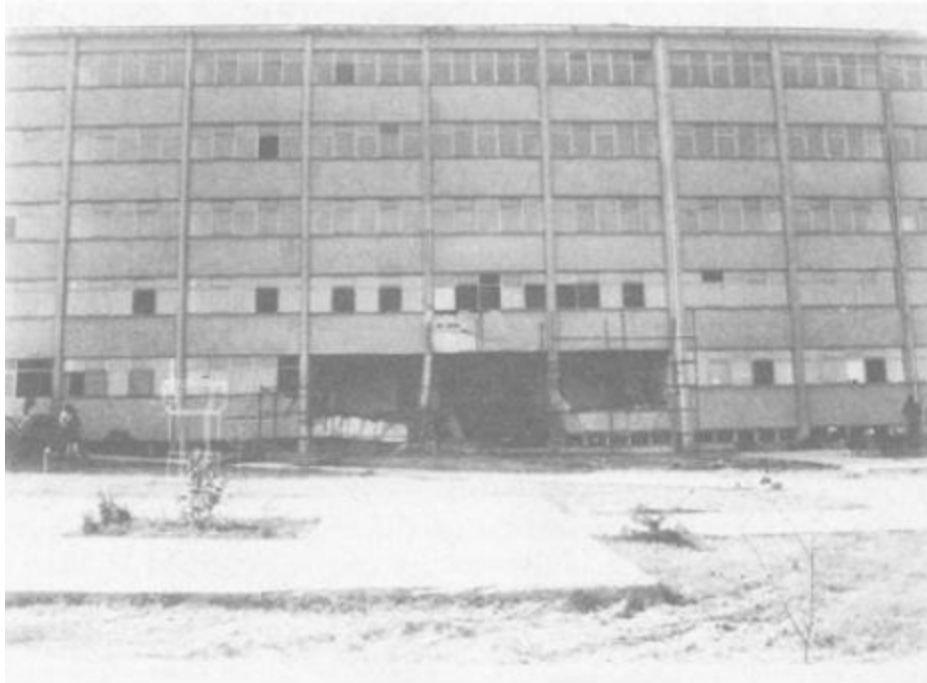
Figure 2-4. Front View of Reinforced Concrete Building Damaged by System Boiler Explosion (Sucuoglu et al., 1994).
