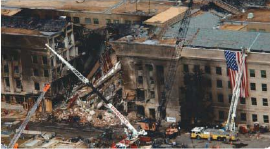
Figure 2-3. Pentagon building after the crash damage (Mlakar et al., 2003)
