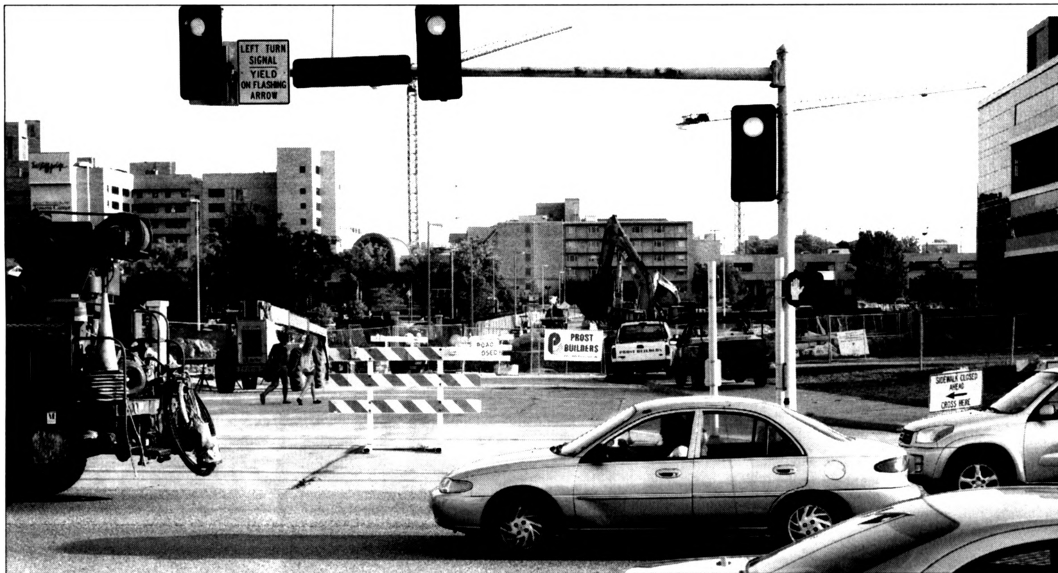
CLOSED FOR REPAIR Major construction on Monk Drive, which connects Stadium Boulevard and Hospital Drive, has forced the closure of the VA Hospital parking lot, which typically serves Tiger fans on game day. However, a temporary drive will provide easy access to a parking lot at Stadium and College.
