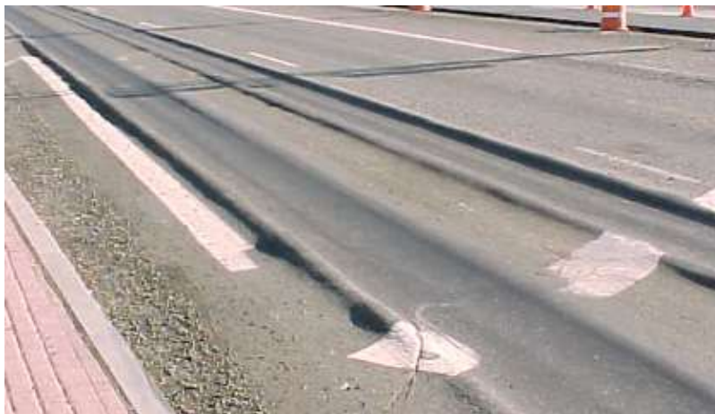
Figure 1. Image of Severe in Field Asphalt Pavement Rutting
